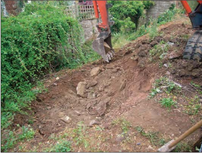
Plate 5 Mechanical ground excavation work commences at the southern end of the site, looking north-west
