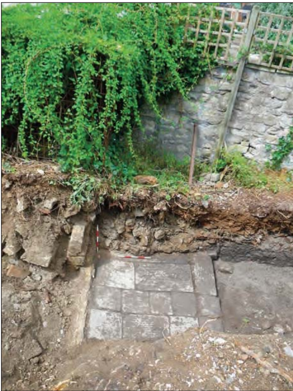
Plate 7 Looking west at structural remains belonging to one of the former terraced houses of Williams' Place. Left of the Pennant flagstone surface (103) is the remains of the north exterior wall of one of the houses (wall 104), while to the right is the buried garden soil 102
