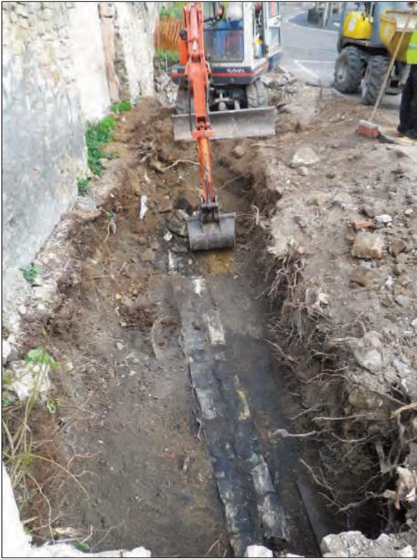
Plate 13 Excavation work in progress north of wall 107; late Victorian wall 113 can be seen at the base of the trench, looking north
