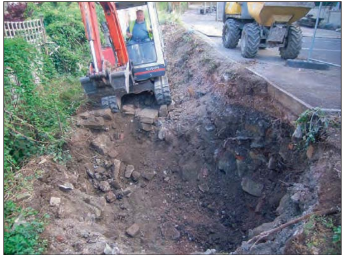
Plate 6 Looking north-east at excavation work in progress at the south-west end of the site
