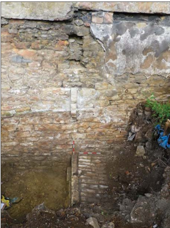
Plate 11 Looking north-west at wall foundation 108 and cobbled floor 109; vestiges of wall 108 can be seen bonded into the east-facing elevation of boundary wall 121
