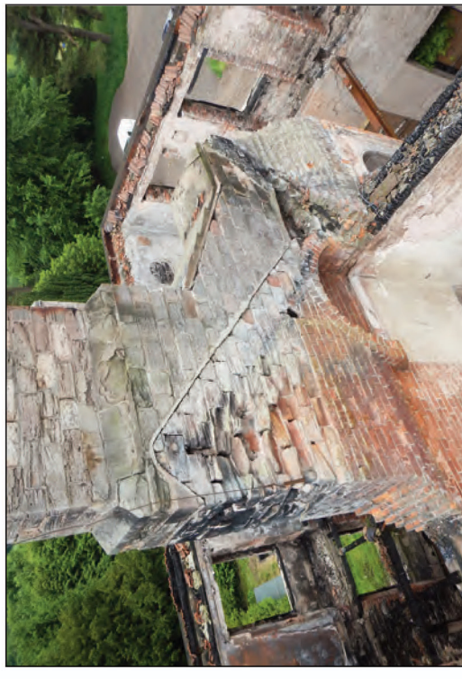
Plate 12 North face of the large chimney stack in the centre of the southern portion of the house, looking south-west
