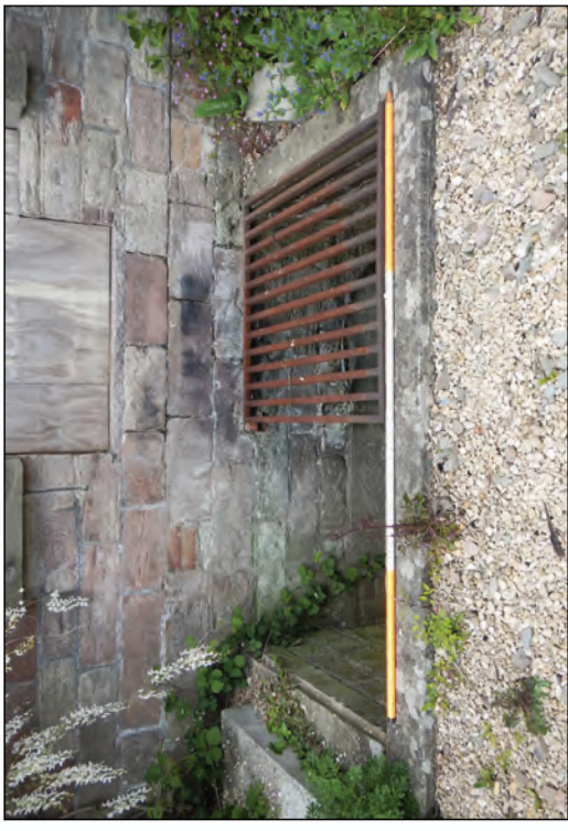
Plate 9 Light-well and access to cellar on south side of the house, looking north
