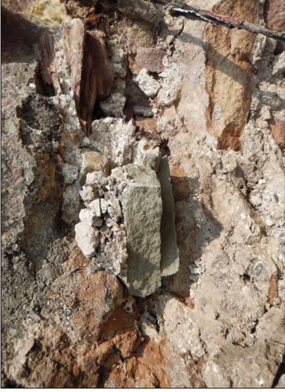
Plate 26 Buff lime mortar in north-south dividing wall of the north wing, looking north
