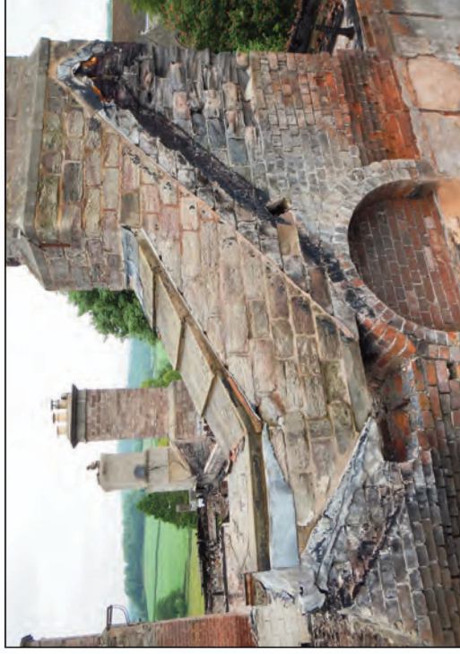
Plate 11 South face of the large chimney stack in the centre of the southern portion of the house, looking north-east
