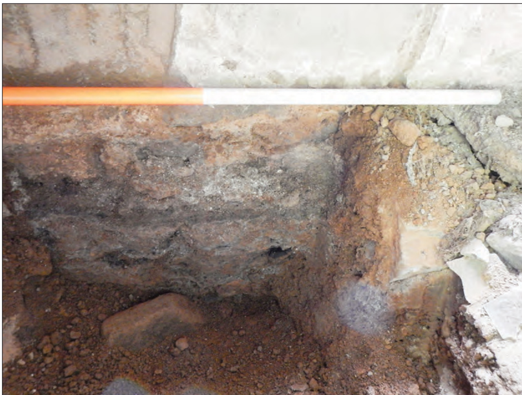
Plate 2 Trial pit 2 west-facing section, foundations and remnant of an earlier floor visible, looking east
