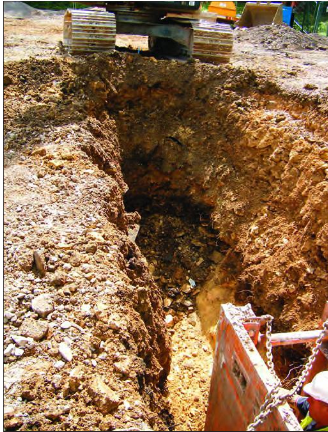
Plate 4 Water main cut by sewer trench
