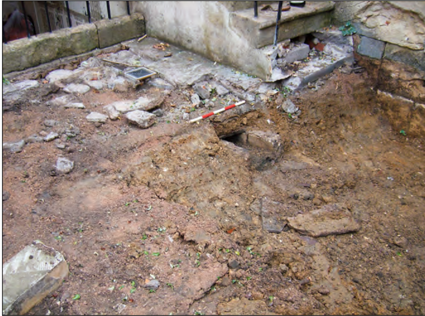
Plate 1 Truncated drain (104), looking towards the stairs up to the house (102), looking west
