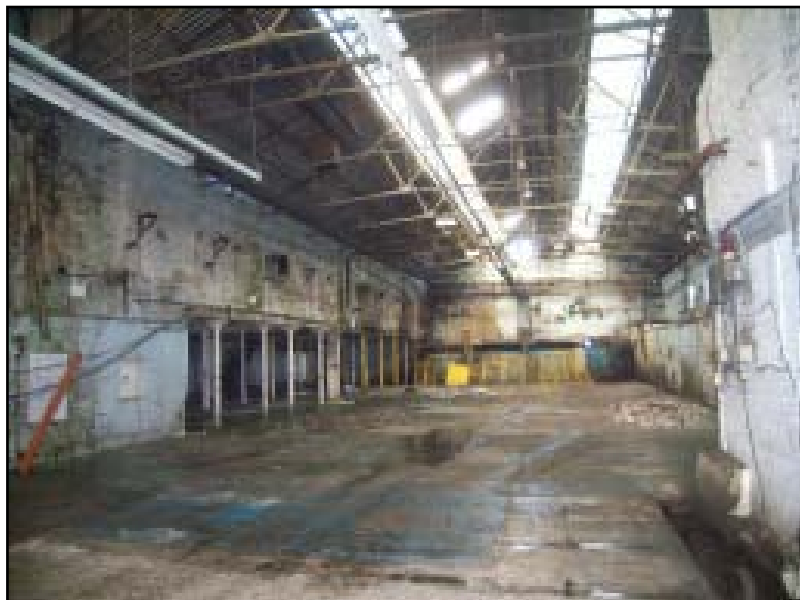
Plate 20 Interior view of the Old Press Shop – looking north. Several trial pits have been broken out, and are awaiting excavation
