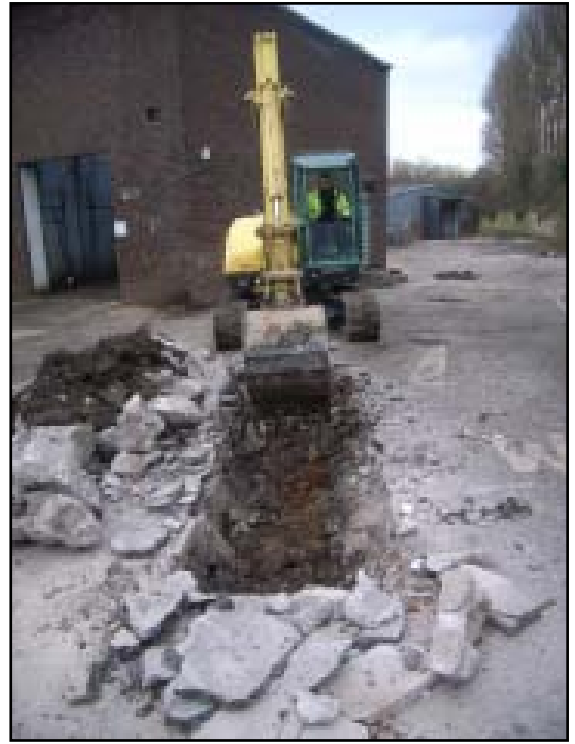
Plate 18 Excavating a trial pit near the south-east corner of the Old Press Shop – looking north-east
