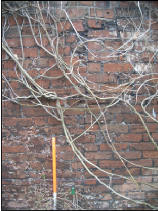
Plate 7 View of the vertical break in the brickwork of the rear elevation, from the south
