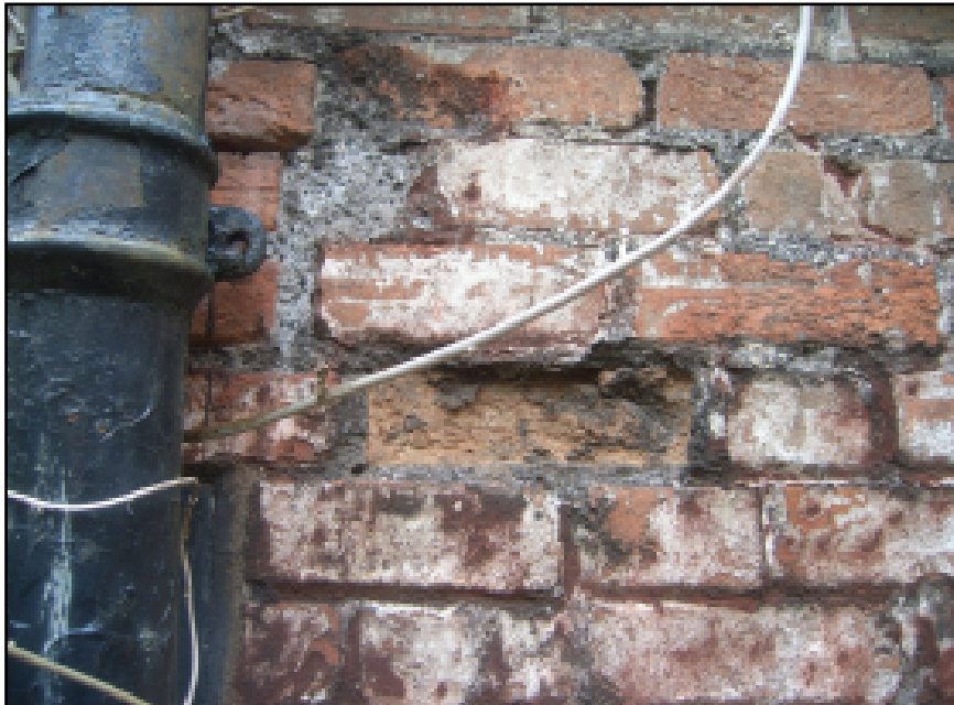
Plate 8 View of degraded brick forming the rear elevation, from the south
