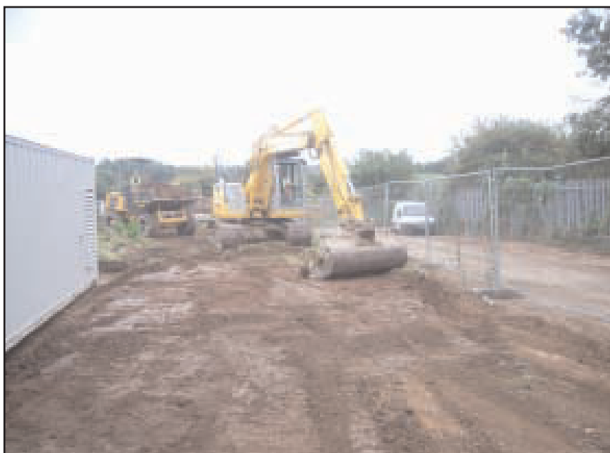
Plate 3 Main site strip commences, next to site cabins (looking south towards River Avon)
