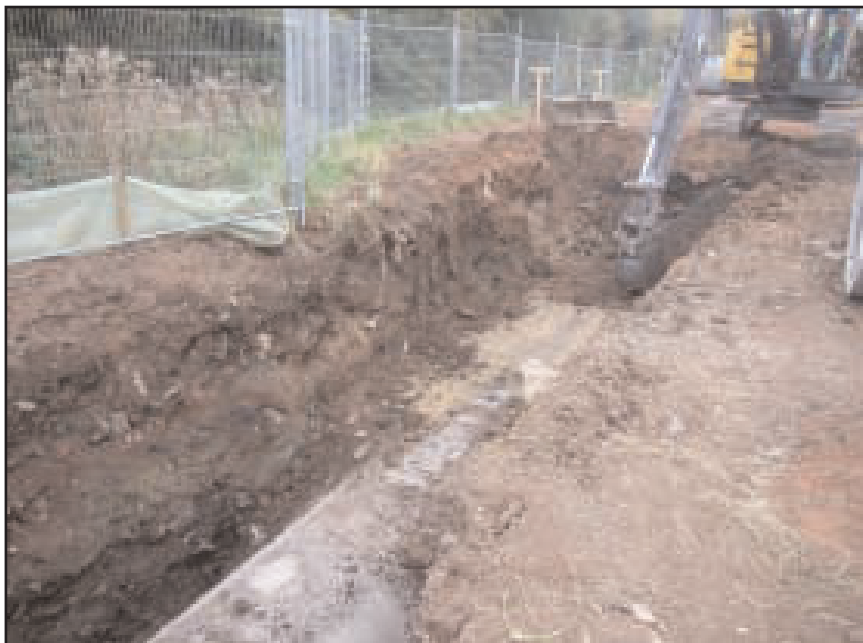
Plate 5 Looking south-west at exposed north-facing section through landfill deposits during excavation of storm-water pipe trench
