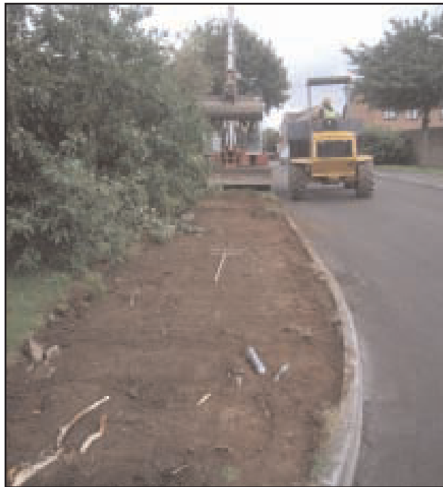
Plate 1 Looking south, next to Myrtle Drive, during topsoil strip of grass verge for new footpath
