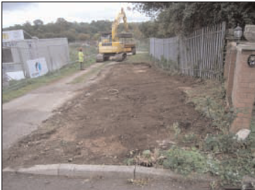
Plate 2 Looking south, during topsoil strip (for road widening) of grass area alongside access track from Myrtle Drive to Myrtle Hall Allotments
