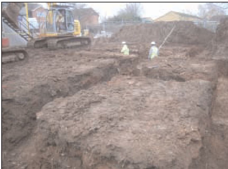
Plate 6 Looking west at the site of 'Building 1' during the excavation of foundation trenches
