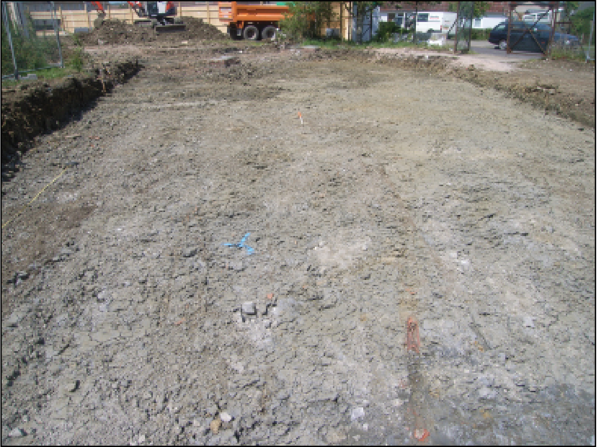
Plate 1 Area A after ground reduction, showing root disturbance and a land drain, looking north
