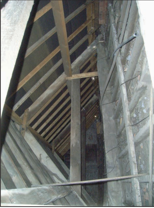
Plate 30 Roof above front part of building, looking east from hatch in former club room
