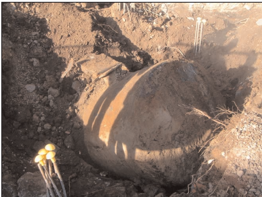
Plate 3 Removal of the diesel tank in area of pile-cap boxes I, K and M
