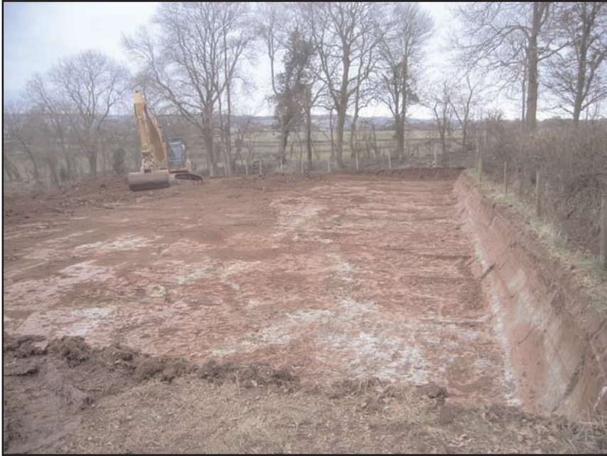
Plate 1 Ground reduction work in progress, looking east, on the site of the proposed agricultural building
