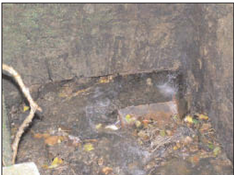
Plate 9 The stone-arched entrance to the culvert in the south-west end wall of the waterwheel pit, looking south-west
