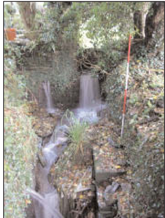
Plate 6 A view along the length of the waterwheel pit showing the offset on the east side with the squared block of sandstone (in front of the base of the ranging pole) on top of the offset, looking north-east (scale 2m)
