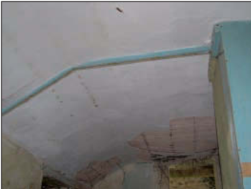
Plate 10 Building A: remains on ceiling of partition dividing the first floor rooms, looking west (no scale)
