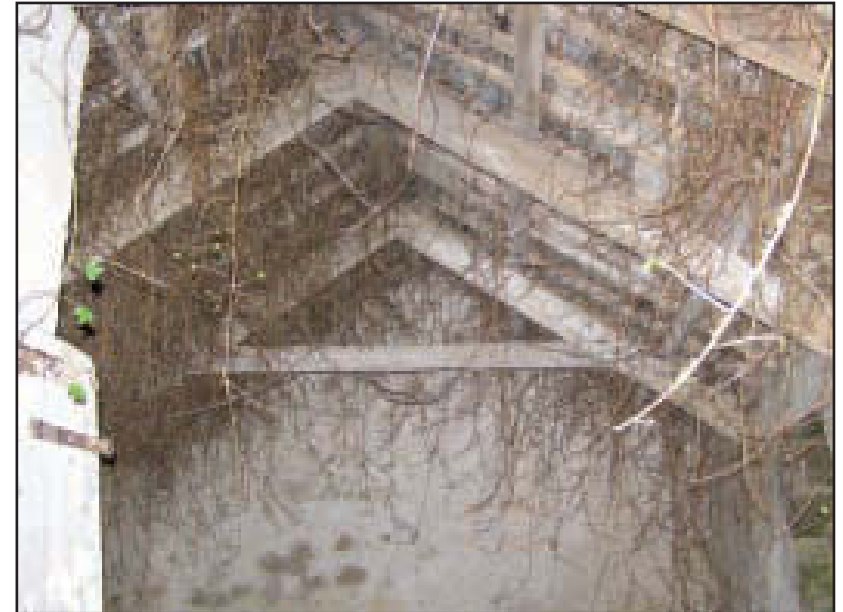
Plate 20 Building D: the roof showing A-frames and purlins, looking east (no scale)
