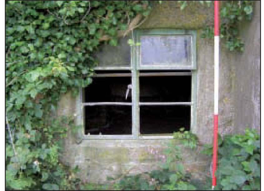
Plate 23 Building D: ground floor window in south elevation, looking north (scale: 2m)
