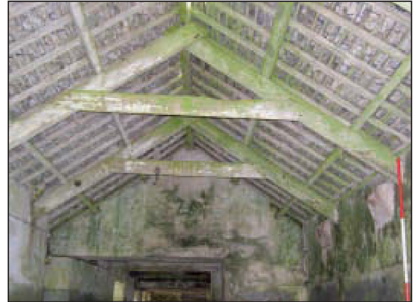
Plate 27 Building E: the roof showing A-frames and purlins, looking west (scale: 2m)
