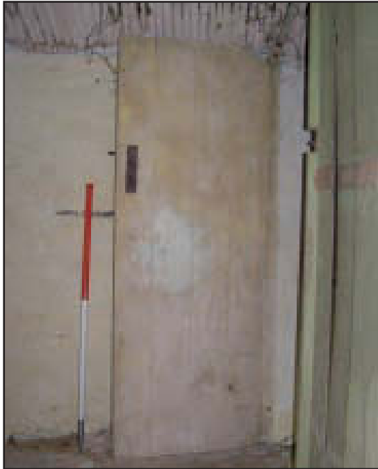
Plate 9 Building A: door from staircase to first floor room, looking north (scale: 1m)
