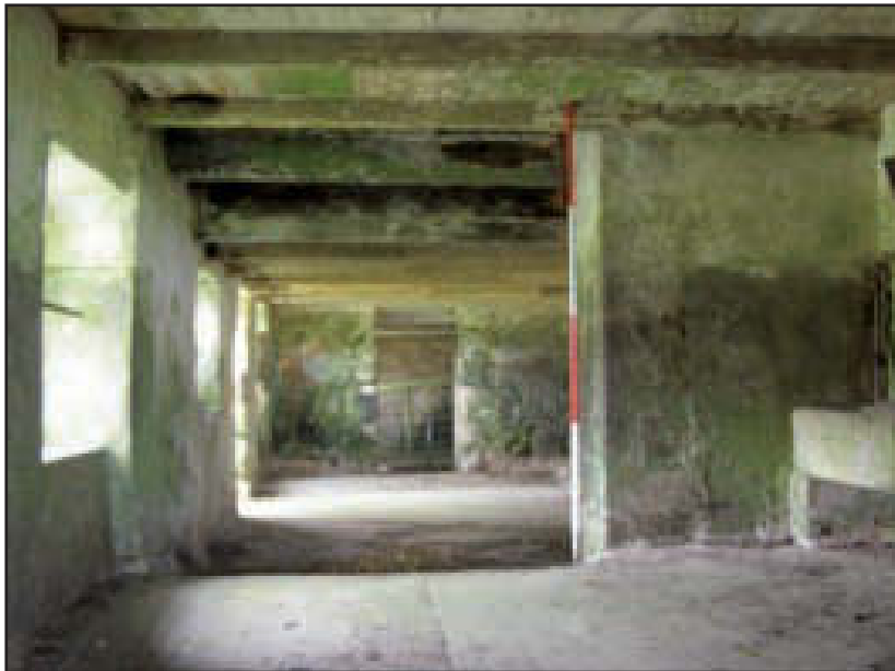
Plate 22 Building D: the doorway between Buildings D and A, looking west (scale: 2m)
