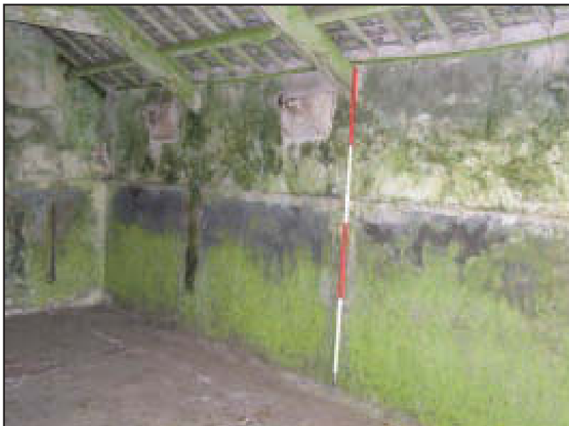
Plate 30 Building E: north wall showing metal covers to ventilation holes and scars caused by the removal of cattle stall partitions, looking north-west (scale: 2m)
