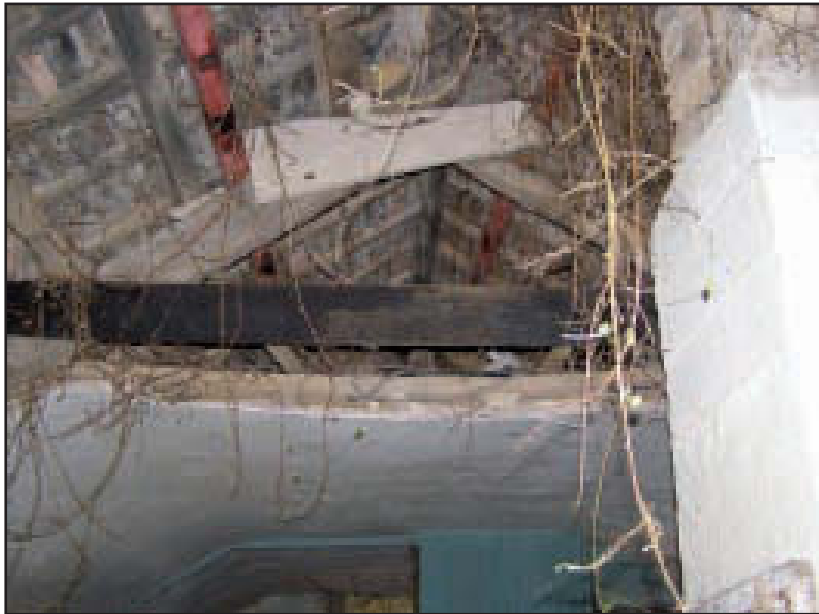
Plate 2 Building A: the roof showing A-frame and lath and plaster ceiling of first floor room, looking west (no scale)
