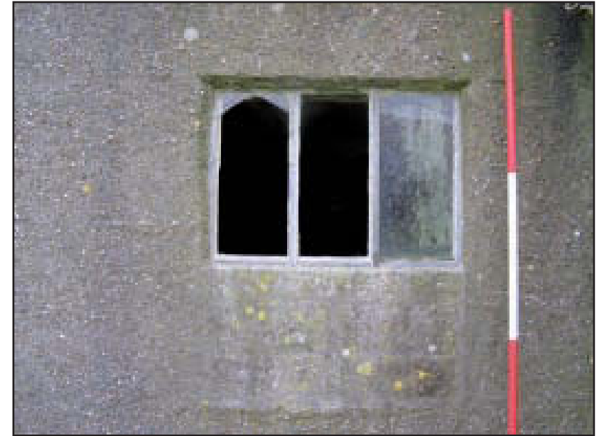
Plate 4 Building A: ground floor window to the west of porch, looking north (scale: 2m)
