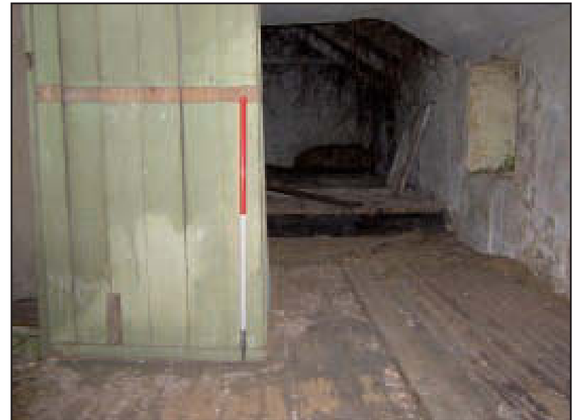
Plate 8 Building A: first floor partition around the head of the staircase, looking east (scale: 1m)
