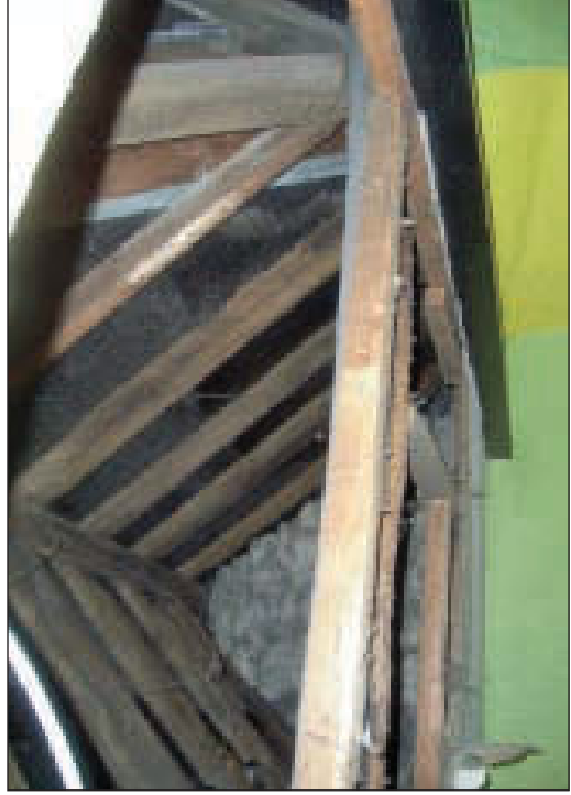
Plate 21 General view across attic space of south-east dormer on north-east side of building, from the south-west
