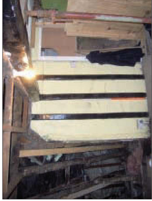
Plate 6 General view of partition separating attic storey from stairwell, from the south-west
