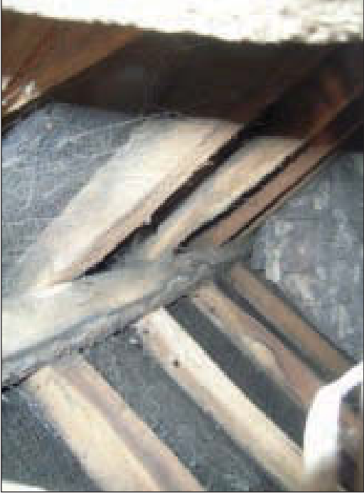
Plate 20 General view across attic space of north-west dormer on south-west side of building, from the north-east
