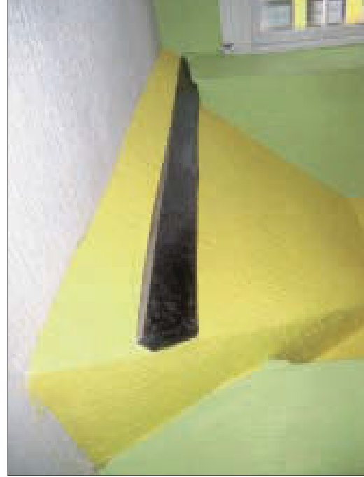
Plate 5 General view of intersection of south-east dormer and main pitched-roof on south-west side of premises, from the north
