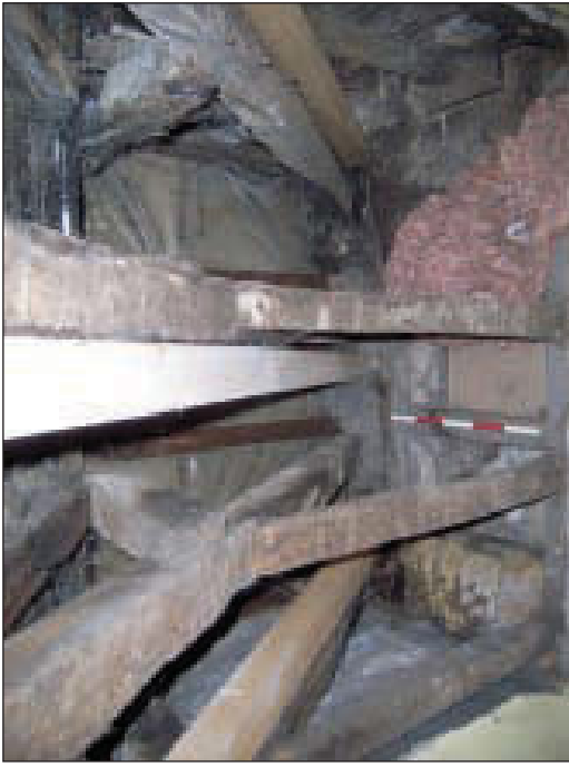
Plate 13 Detail view of lower (eaves) end of exposed structural timbers forming part of the main pitched-roof on the north-east side of the building, from the south-west
