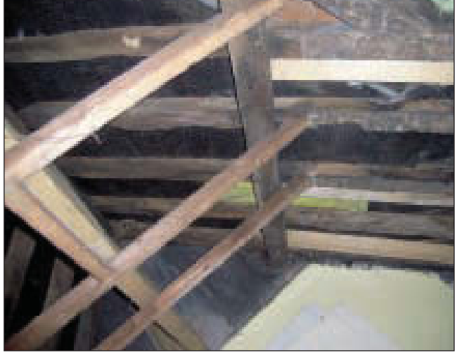
Plate 12 General view of upper (ridge) end of exposed structural timbers forming part of the main pitched-roof on the north-east side of the building, from the south-east
