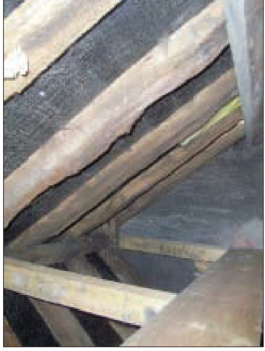
Plate 18 General view across attic space looking towards north-west gable of building, from the south-east
