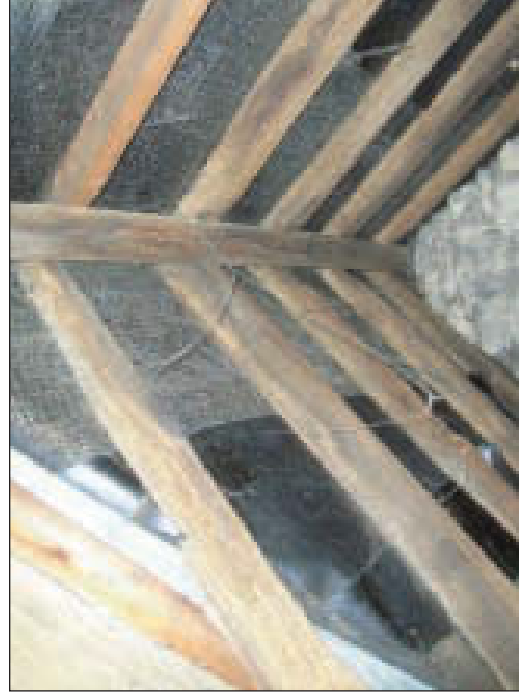
Plate 22 General view across attic space of south-east dormer on north-east side of building, from the south-west
