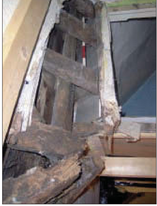
Plate 17 Detail view of timber element to be replaced above door opening leading from attic storey to stairwell, from the south-east
