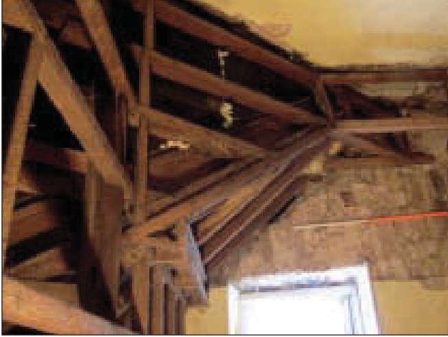
Plate 14 General view of exposed structural timbers to main pitched roof and north-west dormer on south-west side of building, from the north-east
