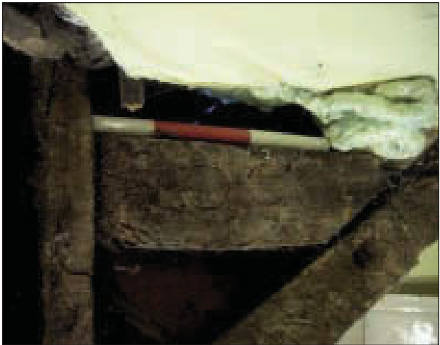
Plate 25 Detail view of structural timber incorporating carpenter's marks on north-east side of building, from the south-east
