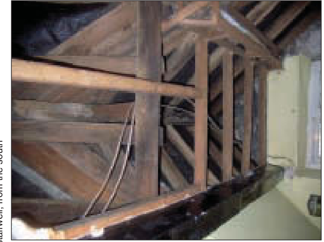
Plate 10 General view of north-west dormer-gable on the south-west side of building, as seen from the attic storey, from the north-east
