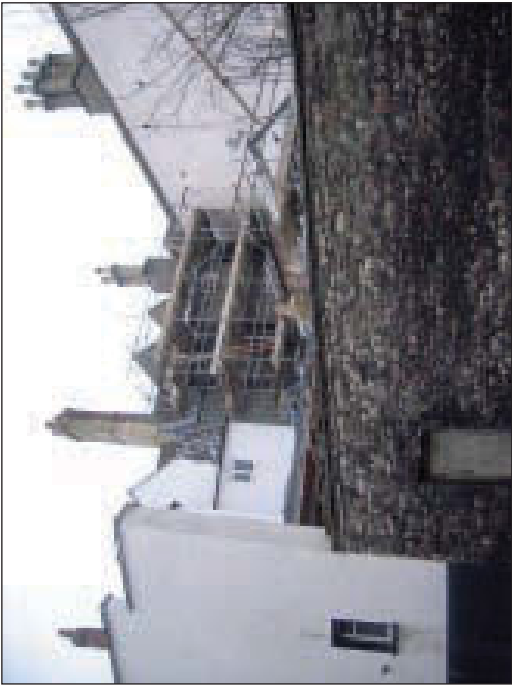
Plate 1 General view of rear (north-east) elevation of the premises, from the east
