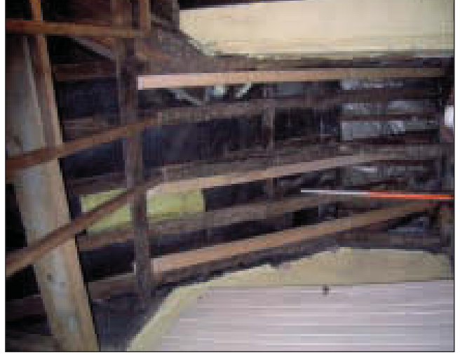
Plate 11 General view of lower (eaves) end of exposed structural timbers forming part of the main pitched-roof on the north-east side of the building, from the south-west
