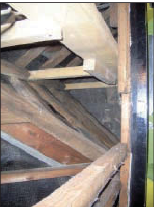
Plate 23 General view across attic space looking towards south-east gable of building, from the north-west
