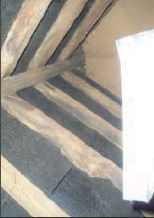
Plate 19 General view across attic space in north-east dormer on north-east side of building, from the south-west
