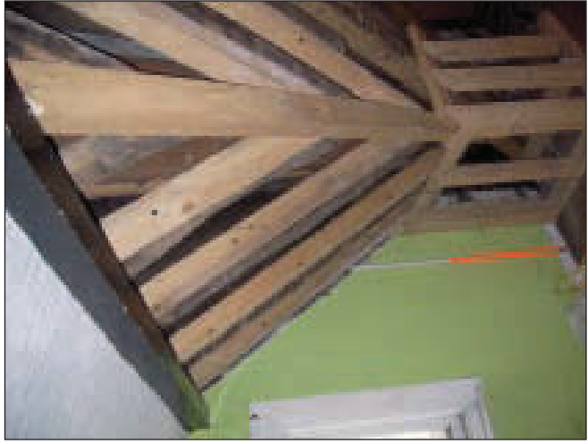
Plate 16 Detail view of exposed structural timbers to main pitched roof and south-east dormer on south-west side of building, from the north-east
