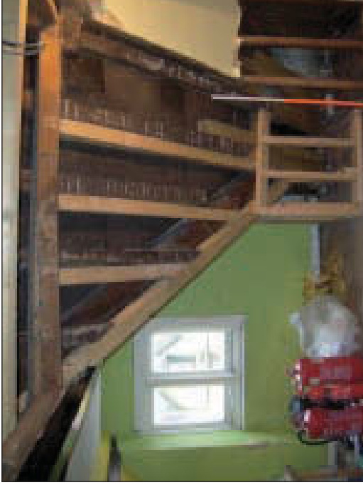
Plate 15 General view of exposed structural timbers to main pitched roof and south-east dormer on south-west side of building, from the north-east
