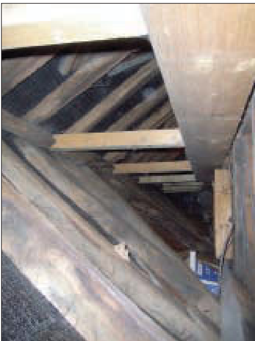
Plate 24 General view across attic space looking towards south-east gable of building, from the north-west
