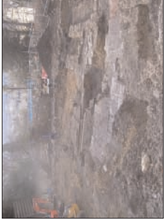
Plate 15 A view of the central and southern areas of the former basement beneath the chapel - looking south
