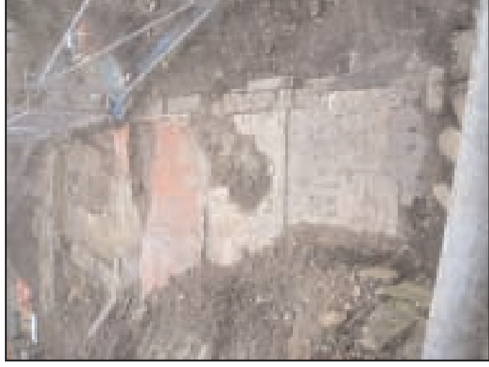
Plate 4 View of extant structural remains at the northern end of the western domestic wing - looking south
