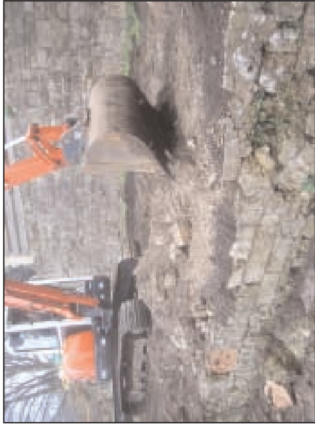
Plate 1 Excavation work in progress within the former NE corner of the basement
