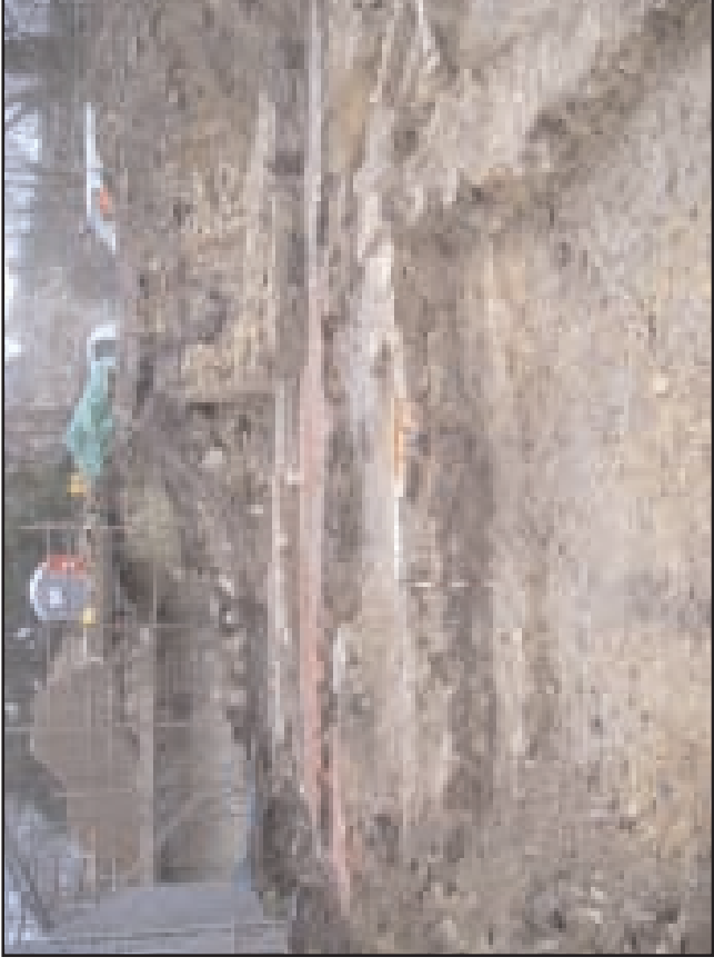
Plate 6 Looking north at south-facing elevation of partition wall 114, which divided Building 'B' from Building 'C'
