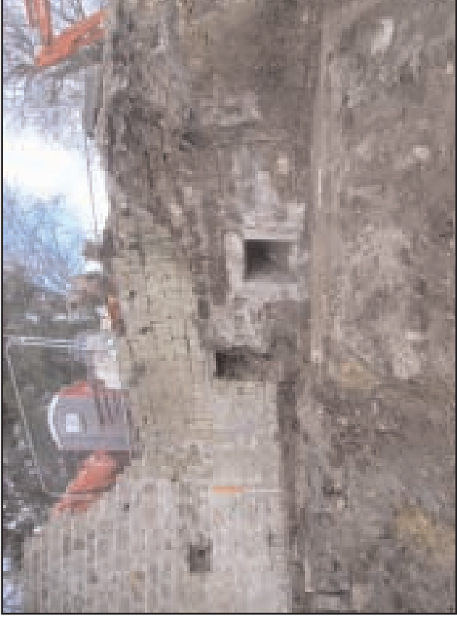
Plate 18 View of the SW-facing (internal) elevation of wall at north end of western domestic wing, showing blocked former coal chutes
