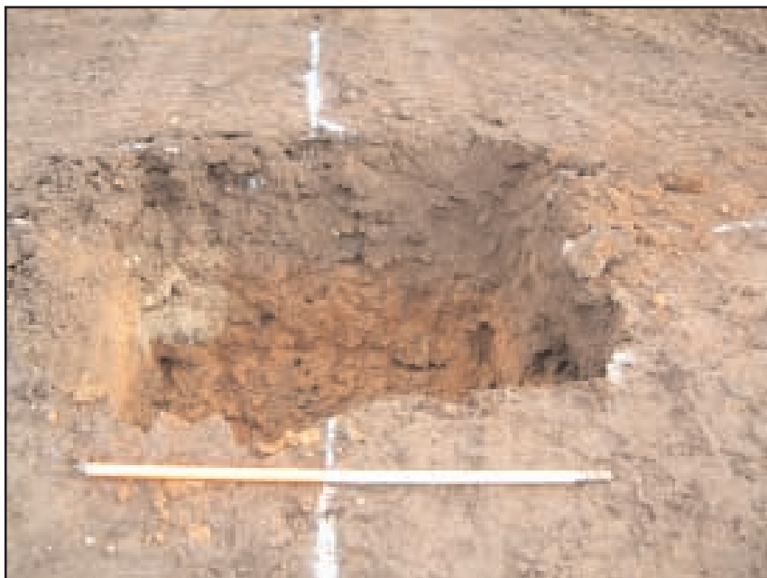
Plate 3 The foundation pit for the climbing frame with the modern intrusion [105] visible in the section, looking east
