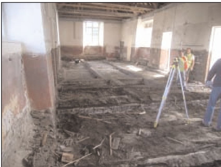
Plate 9 General view of the floor beams in Room G1 after removal of the suspended wooden floor, looking west- south-west
