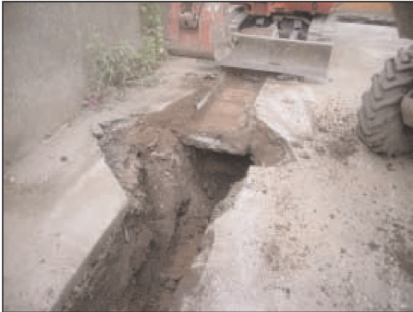
Plate 7 General view of service trench excavation adjacent to Rooms G16 – G18, looking north
