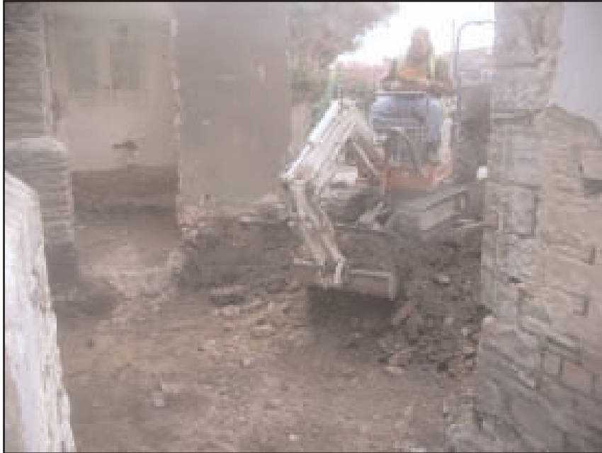
Plate 4 General view of the reduced level excavation between Rooms G1 and G3, looking SSE
