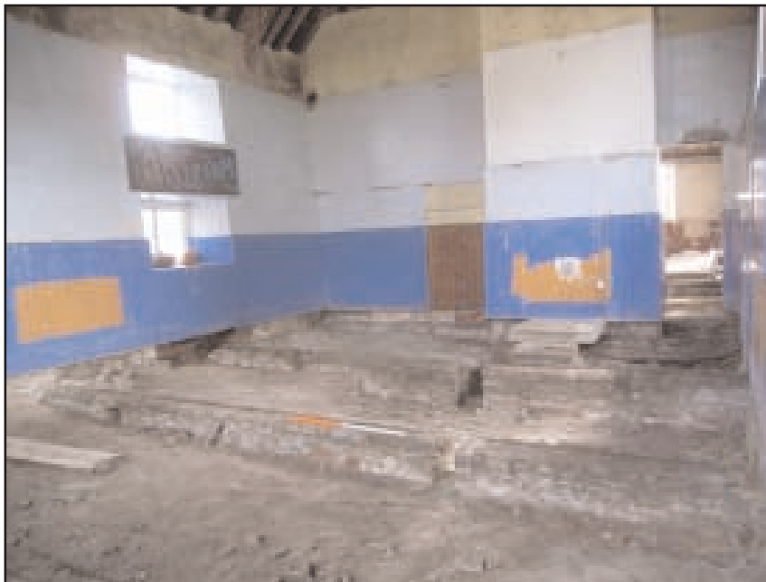
Plate 8 Beams for supporting suspended wooden floor as exposed in Room G2, looking north-east, 1m scale
