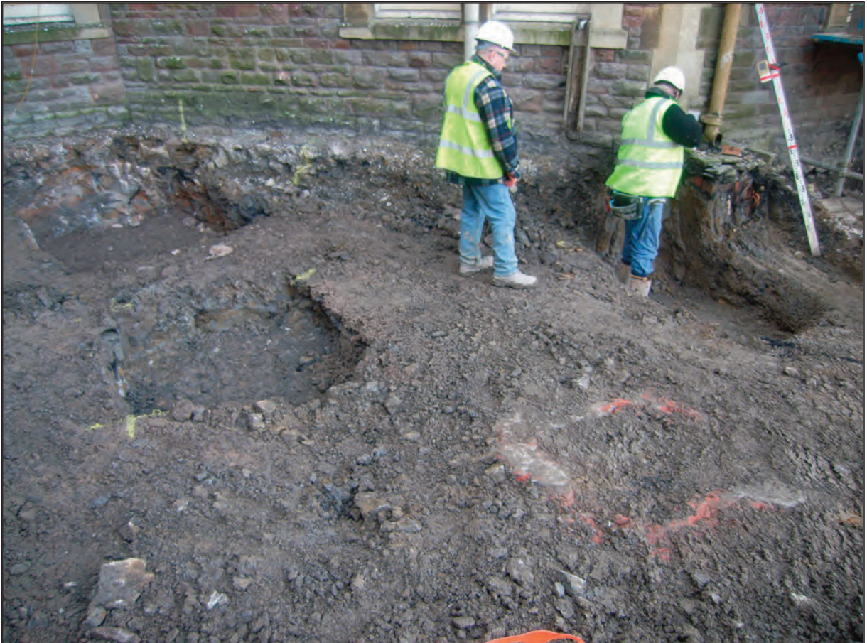
Plate 2 Brick manhole next to the stairwell area of the site, looking west
