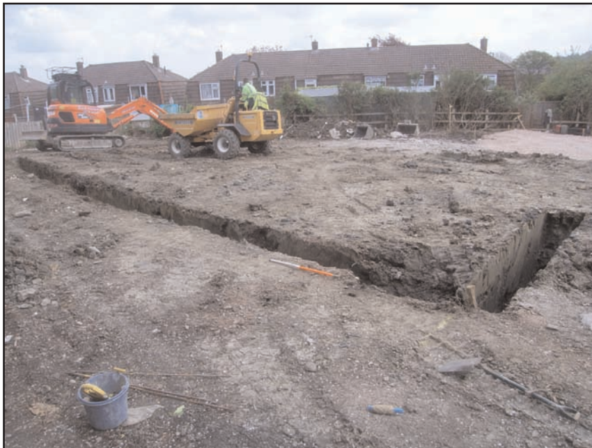
Plate 5 General view of the excavation of footings for Plot B, looking east, 1m scale
