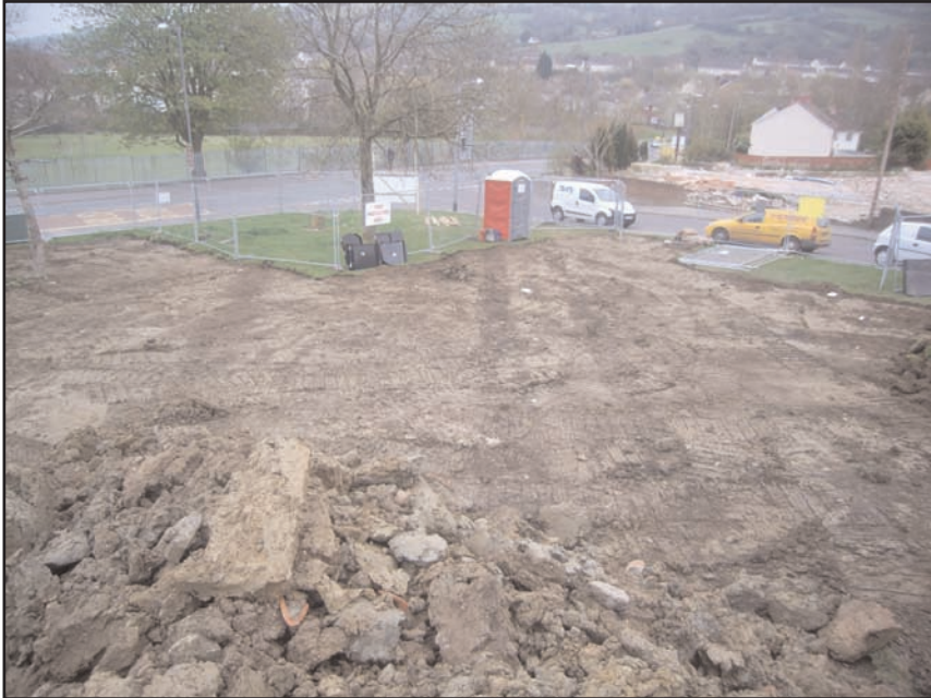
Plate 1 General view of the topsoil strip in the south-east corner of the site, looking south-east
