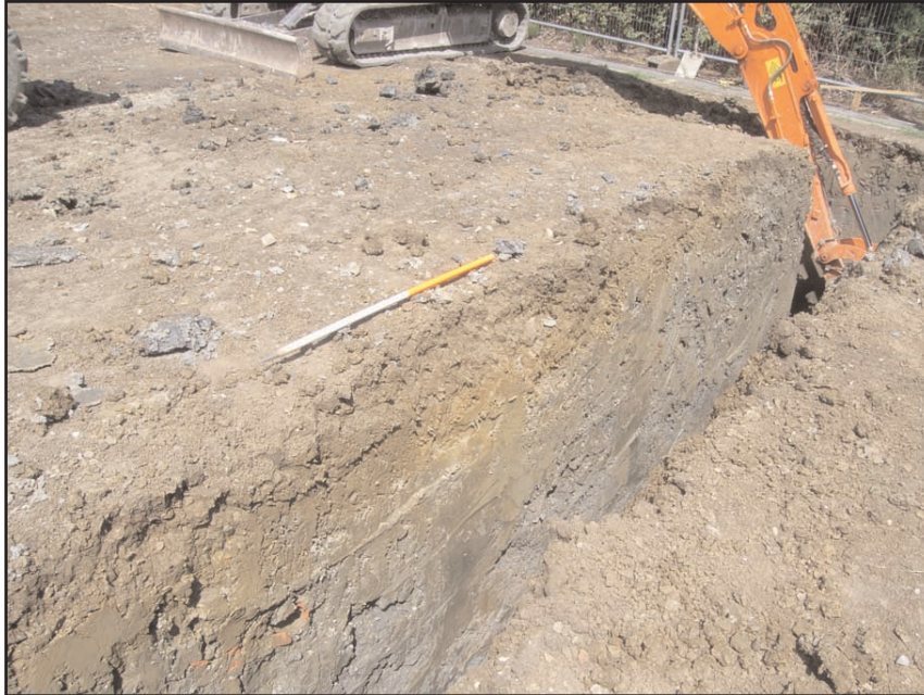
Plate 4 Excavation of the footings for Plot A showing ceramic land drain pipe in section, looking south-west, 1m scale
