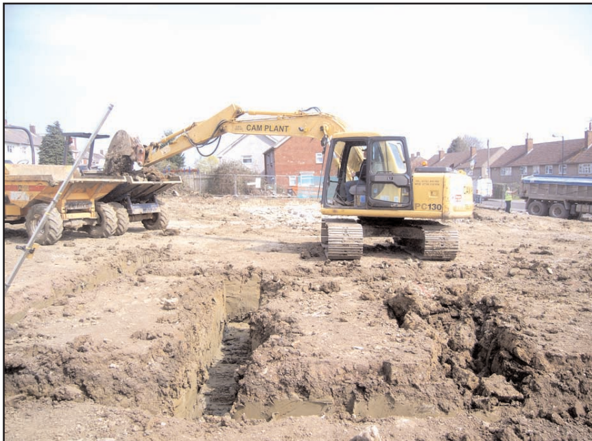
Plate 2 General view of the excavation of footings for Plot D, looking north- north-east
