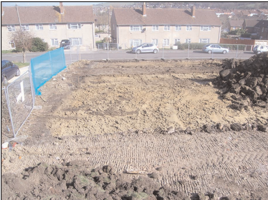
Plate 3 General view of the reduced level excavation around garages 13 and 14, looking west-north- west
