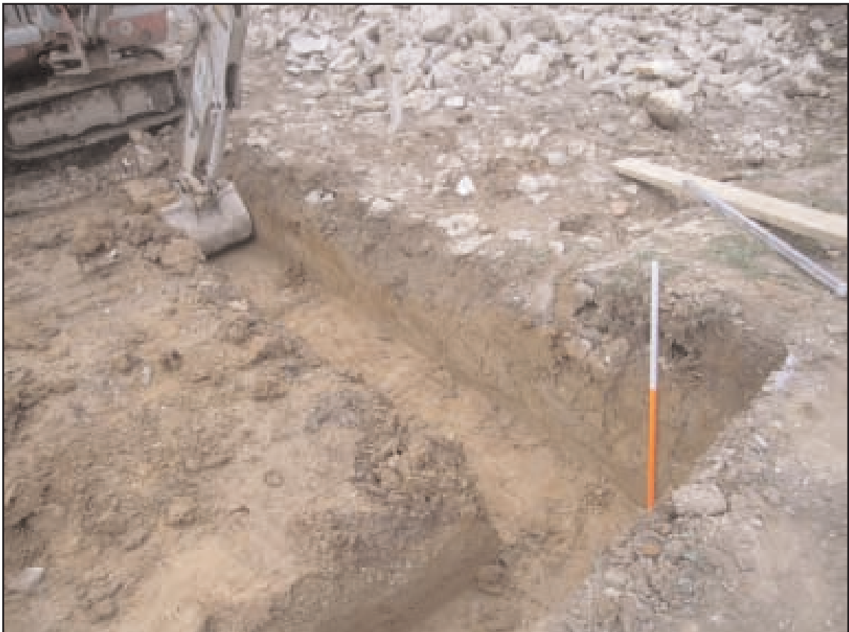
Plate 2 Foundation trench excavation in the south-east corner of the footings, looking north-east, 1m scale
