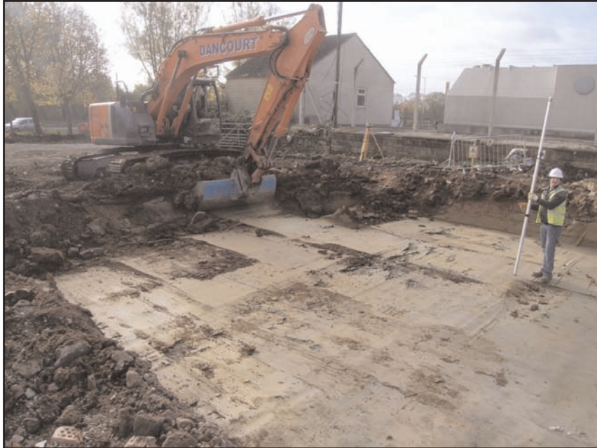
Plate 4 Reduced dig across site of proposed service yard, looking south-west towards electricity sub-station
