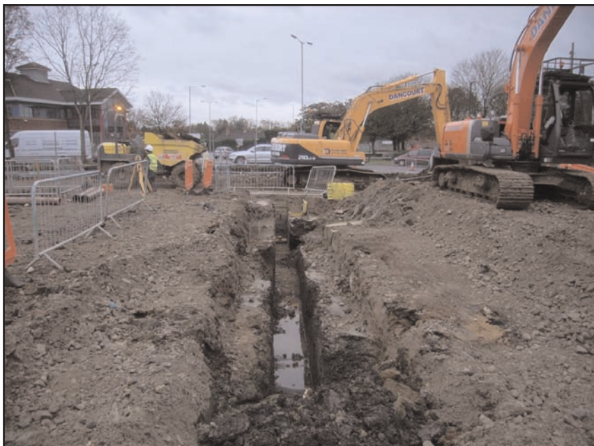
Plate 6 Looking south-east along line of 450mm diameter surface water sewer pipe trench
