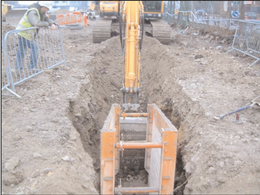
Plate 7 View north-east along route of 300mm diameter surface water sewer pipe trench
