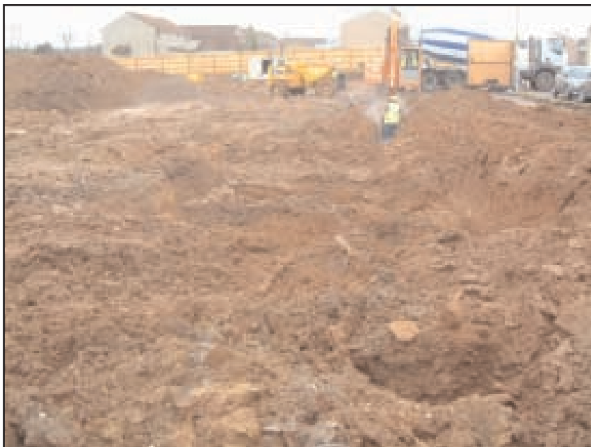
Plate 6 Looking south-east across the site during the excavation of trenches on the site of house plots 1 - 8
