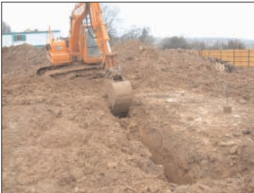
Plate 5 Excavation of a foundation trench on the site of house plots 17 - 20. Looking north
