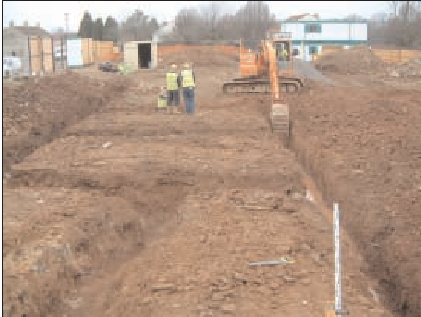
Plate 4 Looking north-west at the excavation of foundation trenches on the site of house plots 9 - 13
