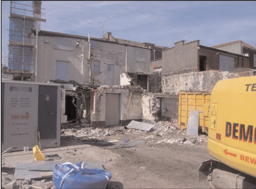
Plate 1 General view of the rear of the Waggon & Horses Public House during demolition, looking north
