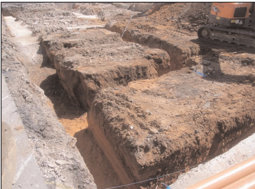
Plate 3 Excavation of foundation trenches in the west of the site, looking east
