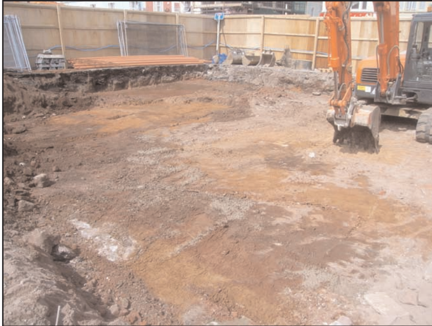
Plate 4 Reduced level excavation of the western side of site, prior to foundation excavation, looking west
