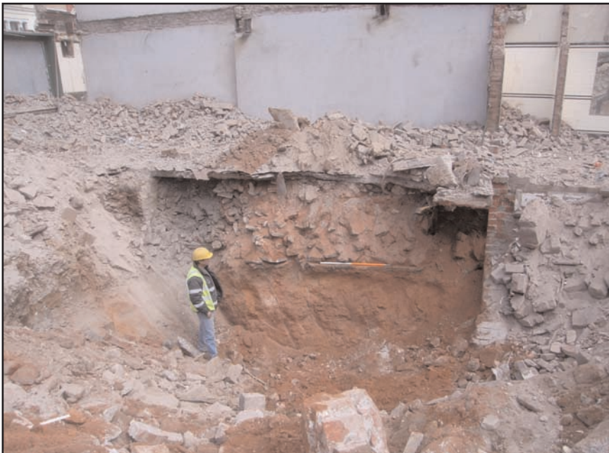
Plate 2 Detail of the main cellar during demolition, also shows the original floor level outside the cellar area and the cellar back- wall continuing to the north-east, 1m scale
