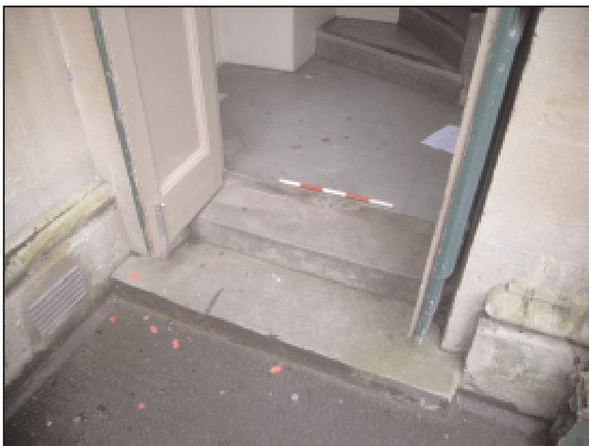
Plate 7 Door to courtyard viewed from outside, showing steps to be altered to form a ramp, looking west-south- west, 0.5m scale
