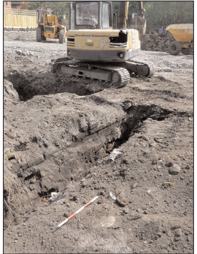
Plate 2 Modern concrete foundations and concrete block wall exposed in the west-facing section of Trench 4, looking south-east, scale 0.5m
