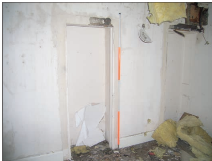
Plate 23 View of blocked-up door opening on south-west wall of Smoking Room on ground floor, from the east
