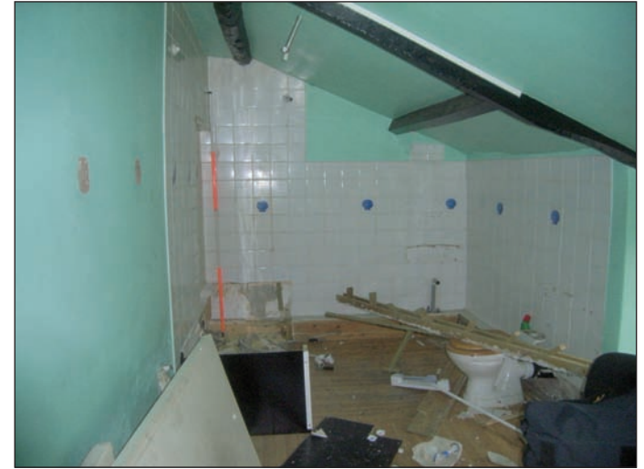
Plate 45 General view across Bathroom on first floor (original Masons Arms), from the south-west
