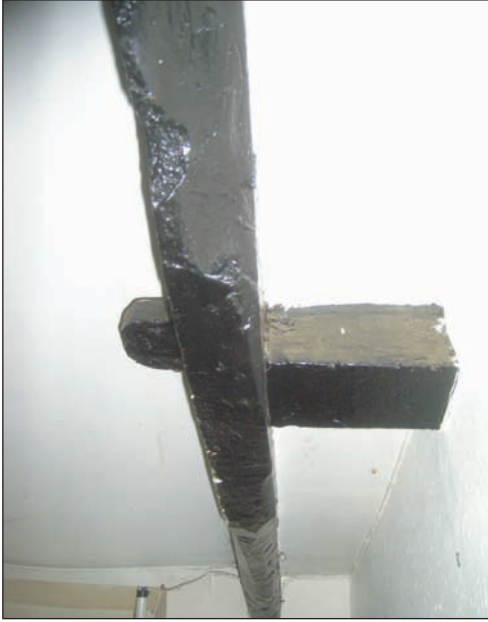
Plate 49 General view of structural roof-timber in Stair Hall on first floor (original Masons Arms), from the north
