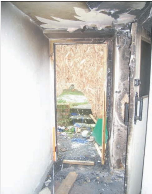
Plate 28 General view across Stair Lobby on ground floor (original Masons Arms), from the north-west
