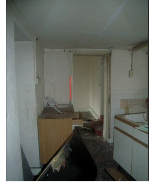
Plate 27 General view across Kitchen on ground floor (original Masons Arms), from the south-west
