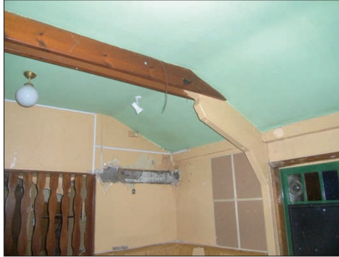
Plate 32 View of portal frame in Public Bar on ground floor (1950s), from the south-west
