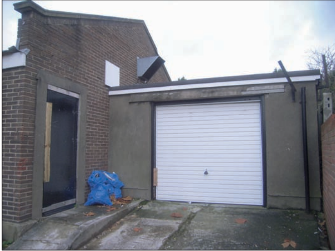
Plate 7 General view of part north-west elevation (1979/80 garage extension) and part south-west elevation (1950s), from the north-west
