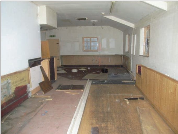
Plate 40 General view across Skittle Alley on ground floor (1950s), from the south-west
