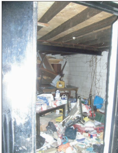
Plate 35 General view across Store on ground floor (early 1970s), from the north-west
