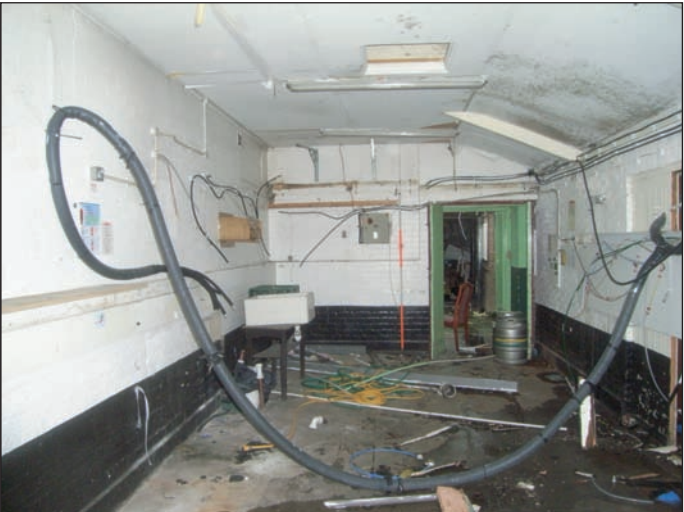
Plate 34 General view across Beer Cellar on ground floor (1950s), from the north-east
