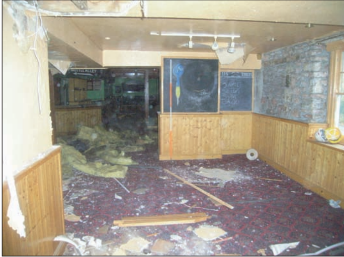
Plate 19 General view across Lounge on ground floor (original Masons Arms), from the north-east
