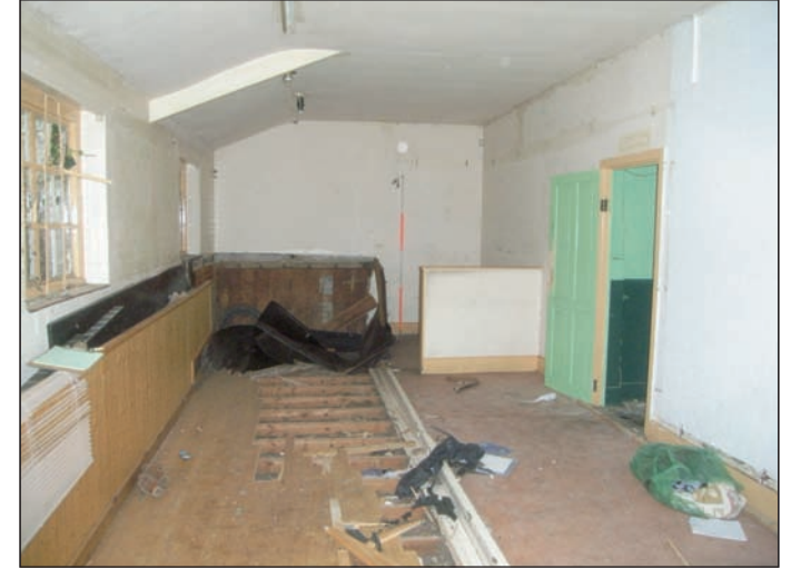
Plate 39 General view across Skittle Alley on ground floor (1950s), from the north-east
