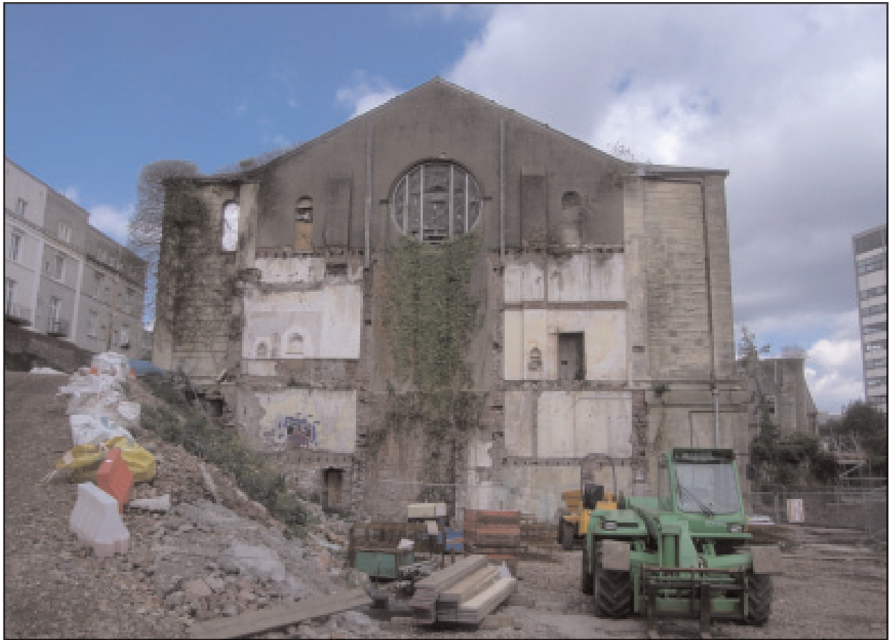
Plate 4 View of the south-west elevation of the cathedral following the demolition of the Presbytery (September 2007)
