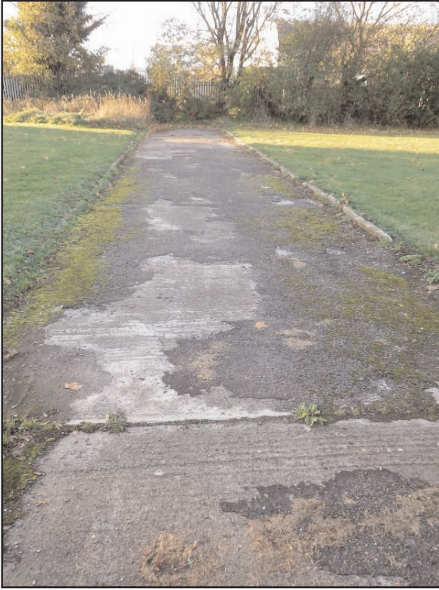
Plate 1 Section of the original road and kerbs of the Balloon Centre, looking west
