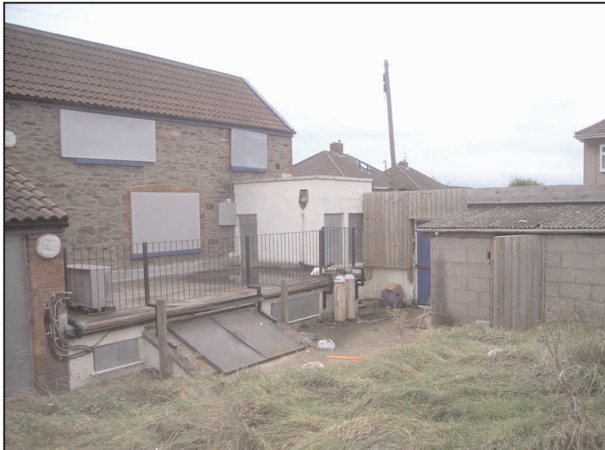
Plate 11 Detail of north-west corner of Lord Rodney showing inspection chamber and 1911 W.C. Extension, looking south- west
