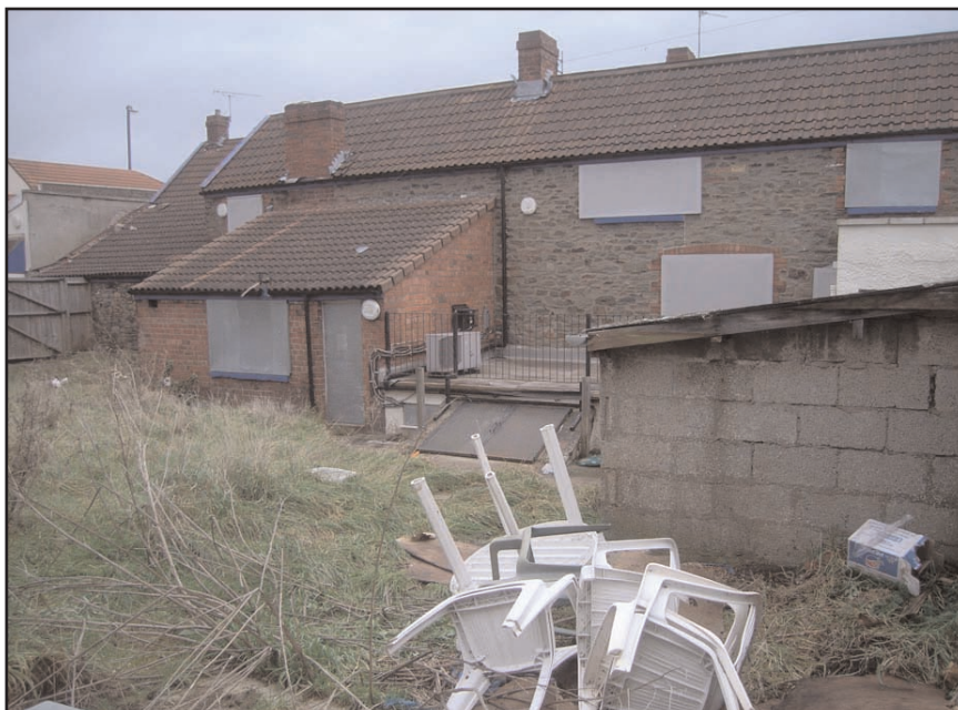
Plate 9 Northern frontage of Lord Rodney showing cellar hatch and 1911 restorations looking south-west from beer garden
