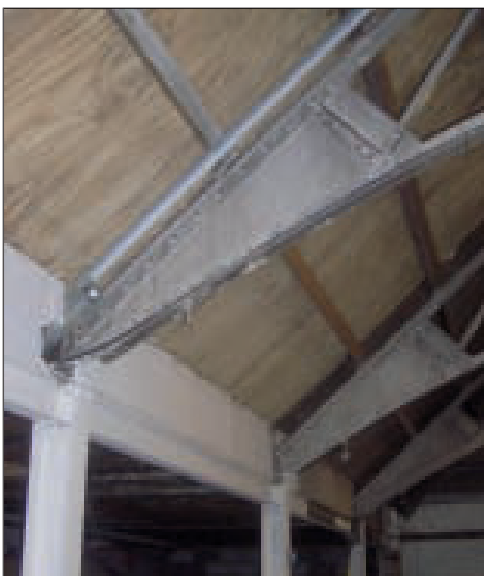
Plate 40 North end of a roof truss of the central block, Room 9, looking north-east
