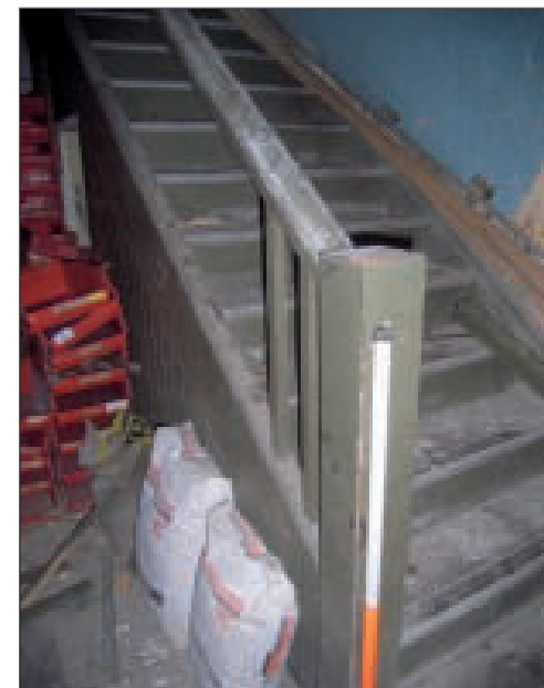
Plate 30 Room 26, staircase in the hallway lead ing to the porch, looking north-east
