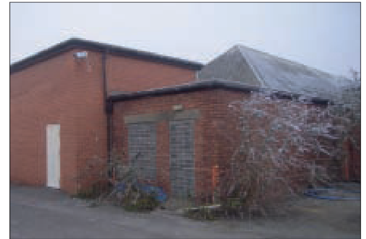
Plate 6 North and east elevations of the English garden wall bond variation block, looking south-west
