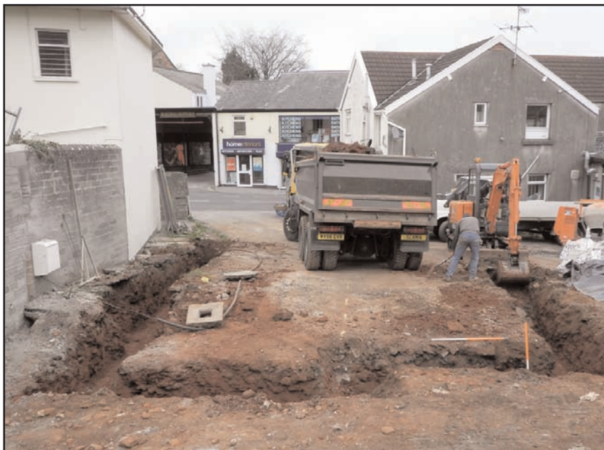
Plate 2 Overall view of work in progress, including initial excavation of Trench 4, looking north-east, scale 0.5m
