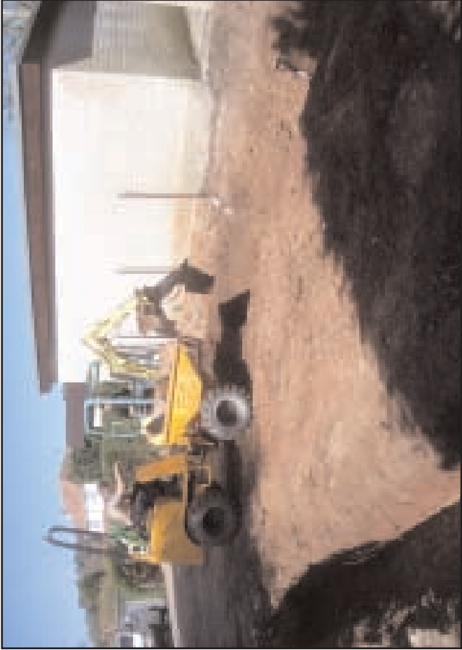
Plate 1 General view of the foundation excavation for the new garage, looking north-west
