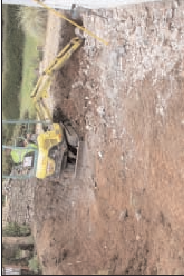
Plate 3 South-facing section of the extension reduced level excavation and foundation excavation, looking north-east, 0.5m scale
