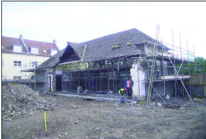
Plate 5 The rear elevation of the Victorian school, after the demolition of an original gabled single-storey extension (as well as two later flat-roofed extensions)
