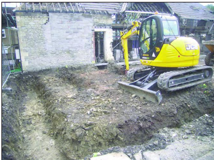
Plate 6 Foundation trench excavations in progress near the north-west corner of the original building
