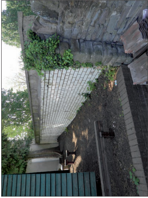
Plate 16 Tiles of original girls' latrine block within northern precinct wall, looking north-west
