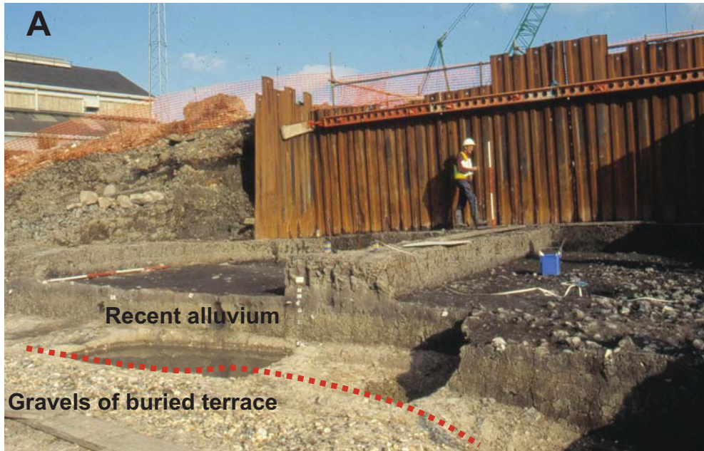
Figure 15. A: Buried terrace of the Medway lying beneath recent alluvium at the Medway Tunnel site. B: fluvial sands and gravels overlying chalk at Cuxton.
