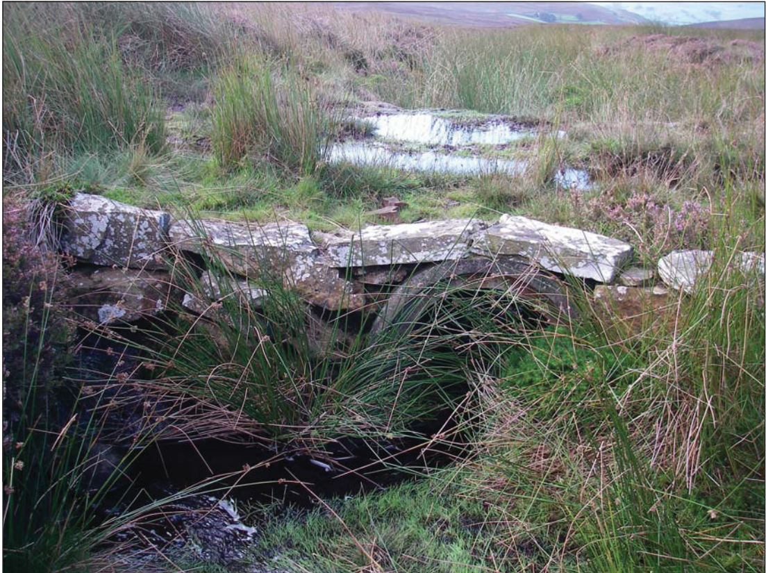
Plate 7. Modern culvert under the existing track along the northern section of the proposed route, looking south-west
