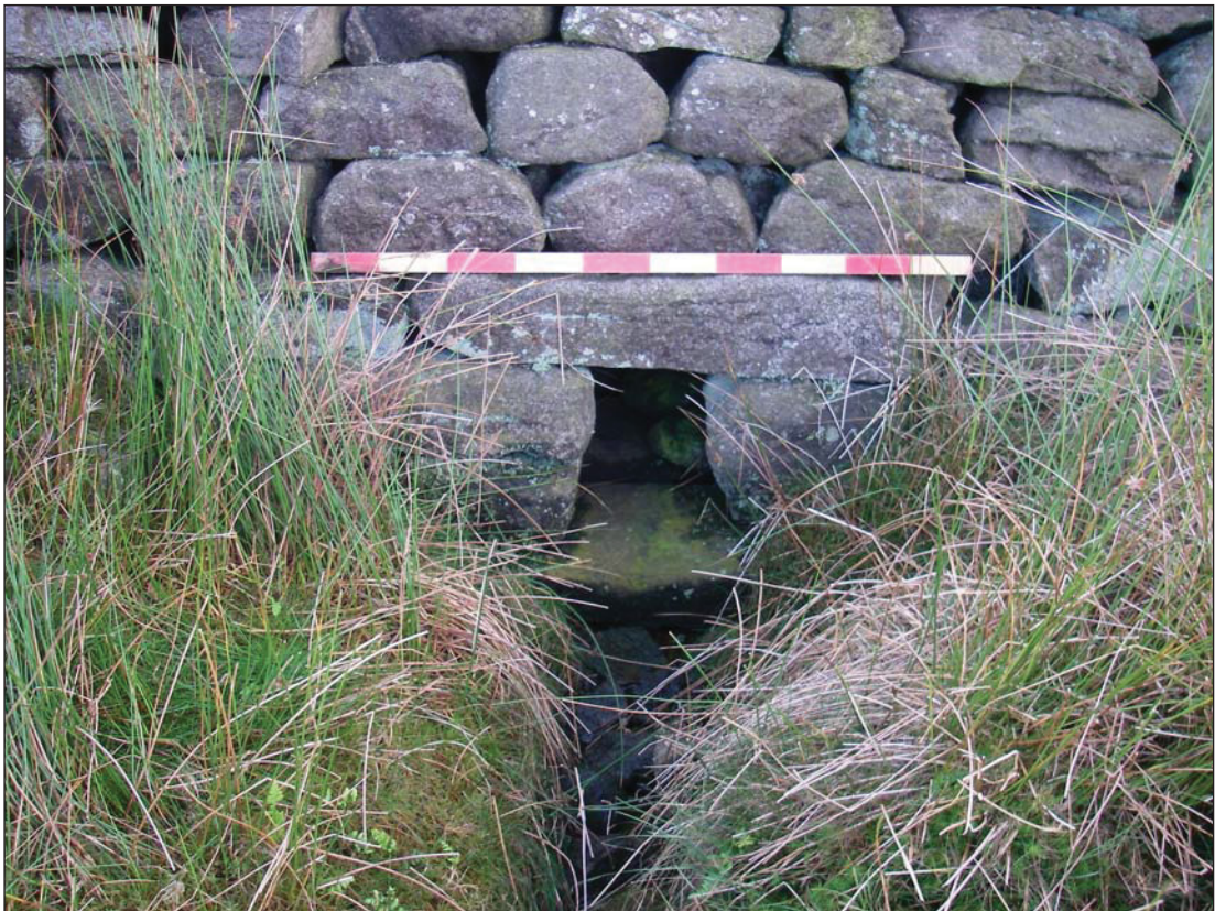
Plate 6. Culvert in the base of the eastern side of the dry stone wall, close to the southern end of the proposed route of the track
