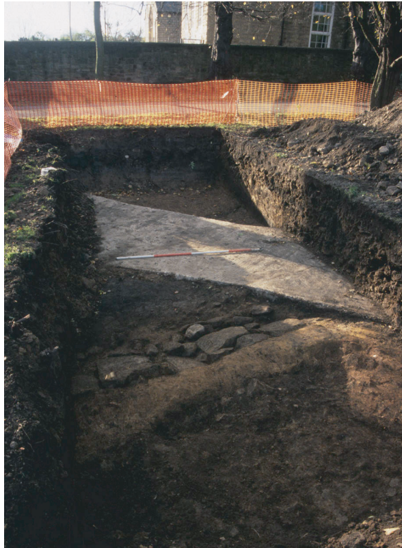
Plate 3. Trench 4, moat retaining wall (1096) visible in the foreground, and the concrete base (1084), looking south-west
