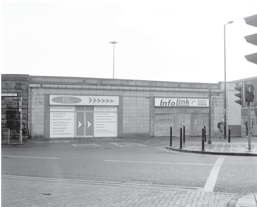
6 9716/11 E Shop frontages obscuring detail of viaduct on south-west elevation
