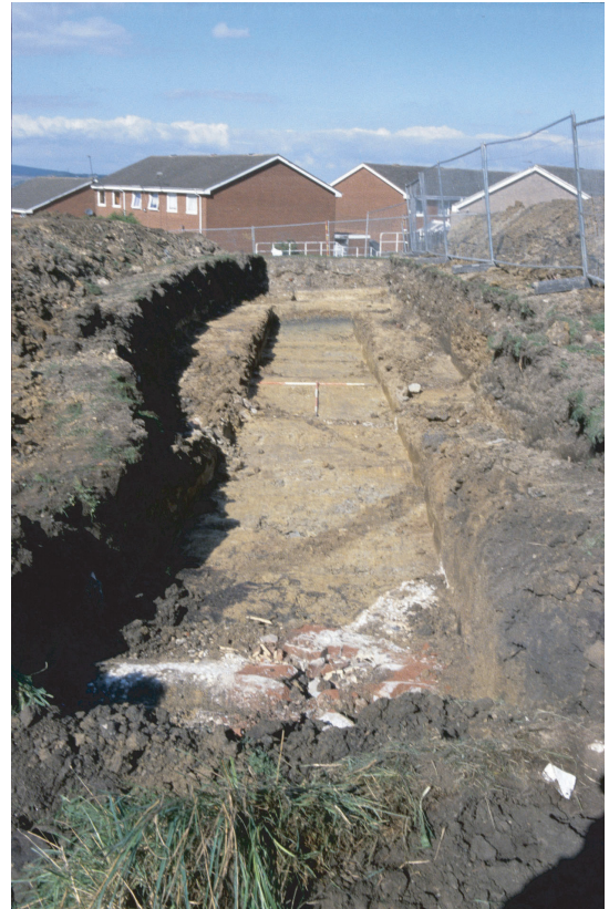
Plate 4. Trench 9, general trench shot showing modern disturbance and field drains, looking north
