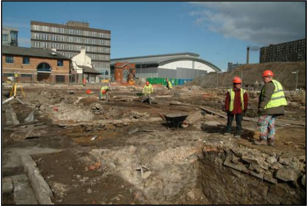
Plate 5: excavation of buildings 1-7 showing gennel between buildings 6 and 7 in the foreground. View north-east
