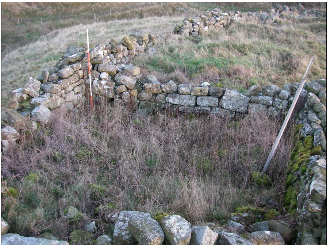
Plate 20. The remains of a building or sheep pen, in the eastern building range nearest to Ironhouse Bastle, looking east
