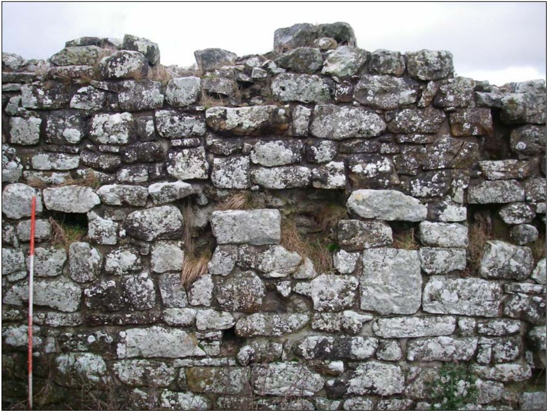
Plate 15. The interior northern wall of the bastle, with a number of beam slots visible
