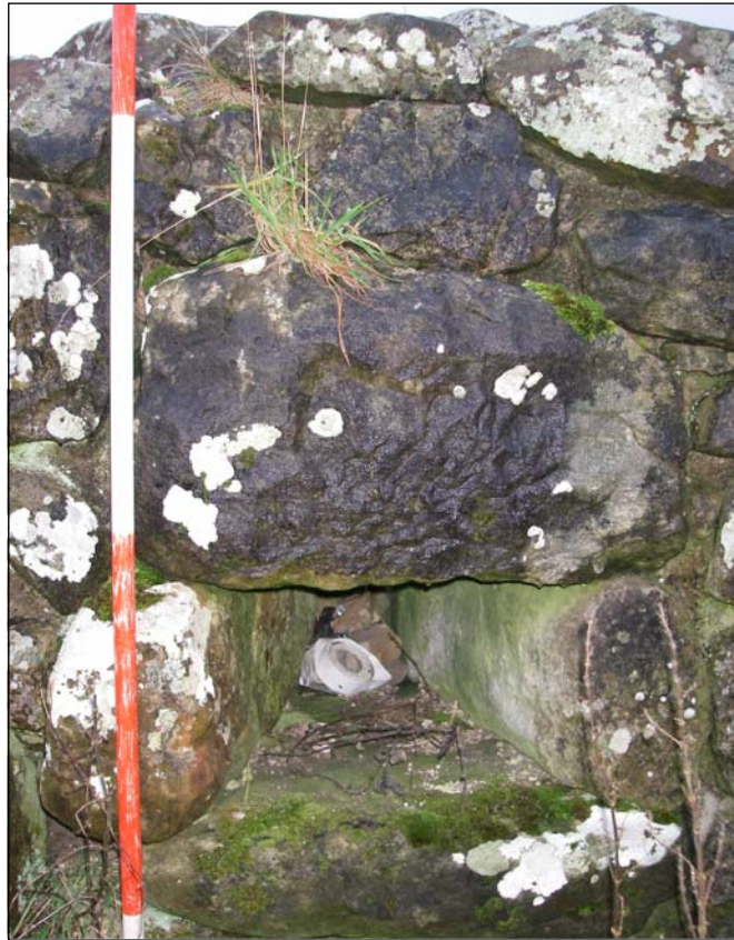
Plate 13. The interior of the slit-vent in the southern wall of the bastle
