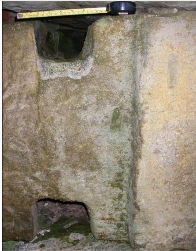
Plate 11. The drawbar tunnel on the northern wall of the bastle doorway to the top, with the hole for the drawbar from the opposing wall below
