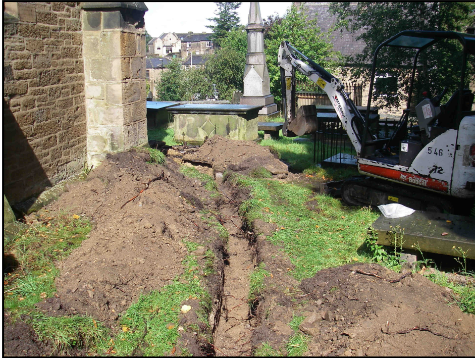
Plate 3. The service trench passing the eastern wall of the church, view north
