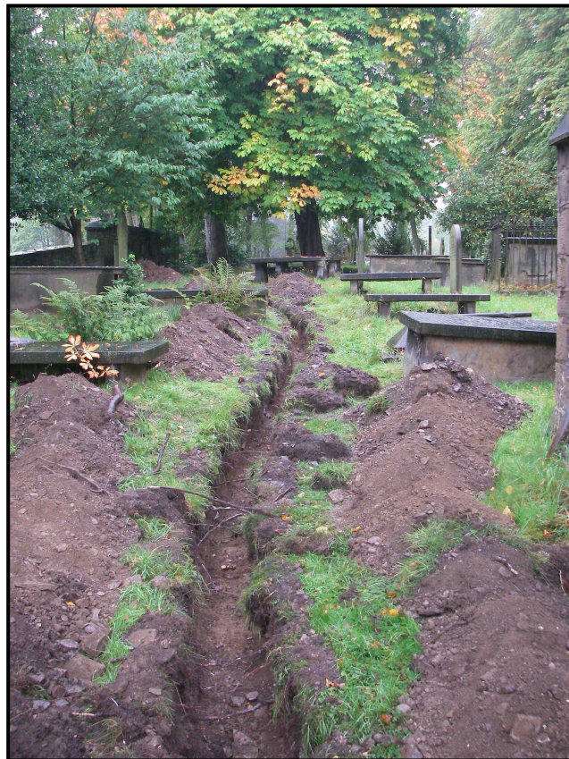
Plate 2. The excavated service trench, view south from the church towards the churchyard gate
