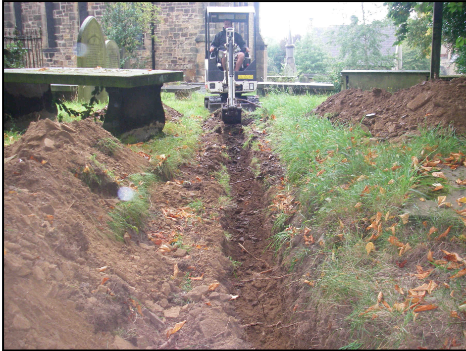
Plate 1. Excavation of the service trench, view north from the churchyard gate towards the church
