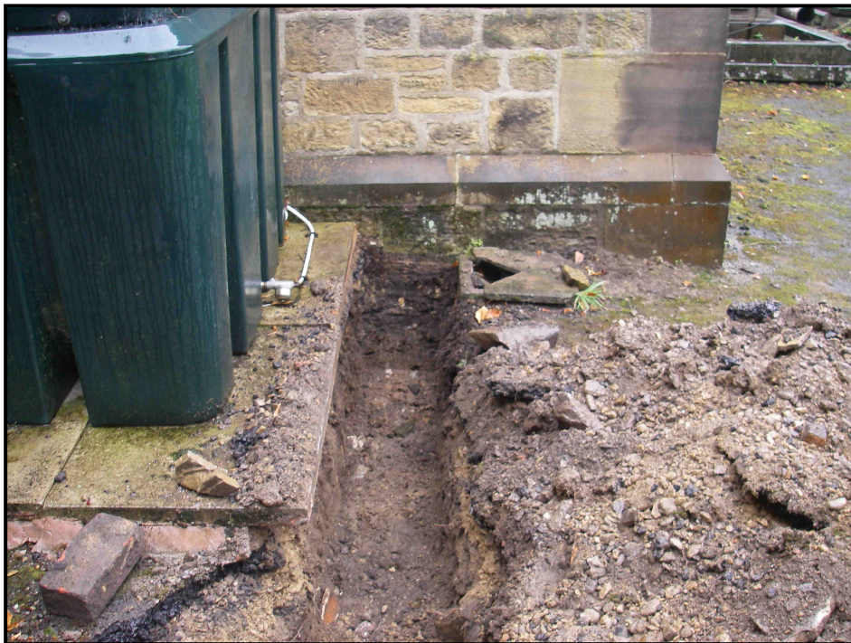
Plate 4. Terminus of the service trench on the church's eastern wall, view west
