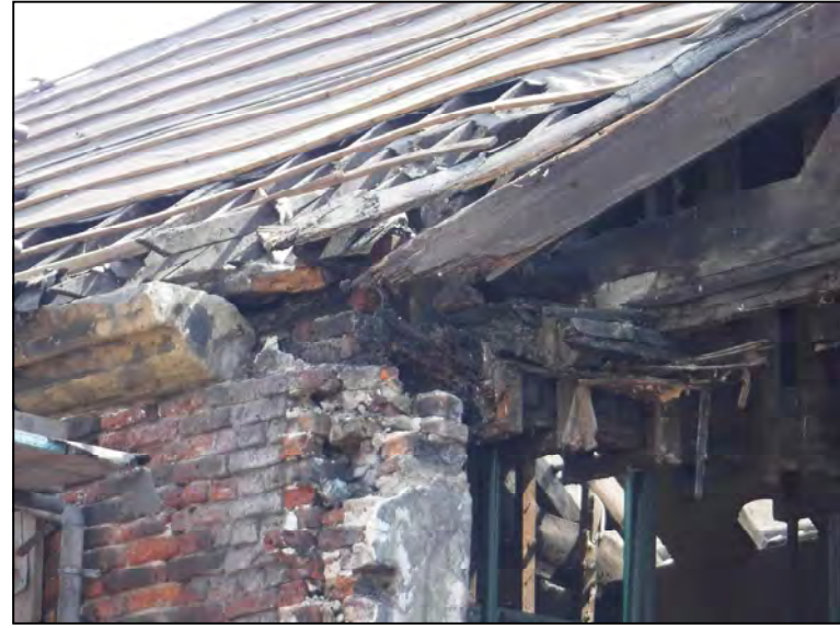
Plate 4. Advanced decay in timbers at join of Trusses 1 and 2, looking north-east
