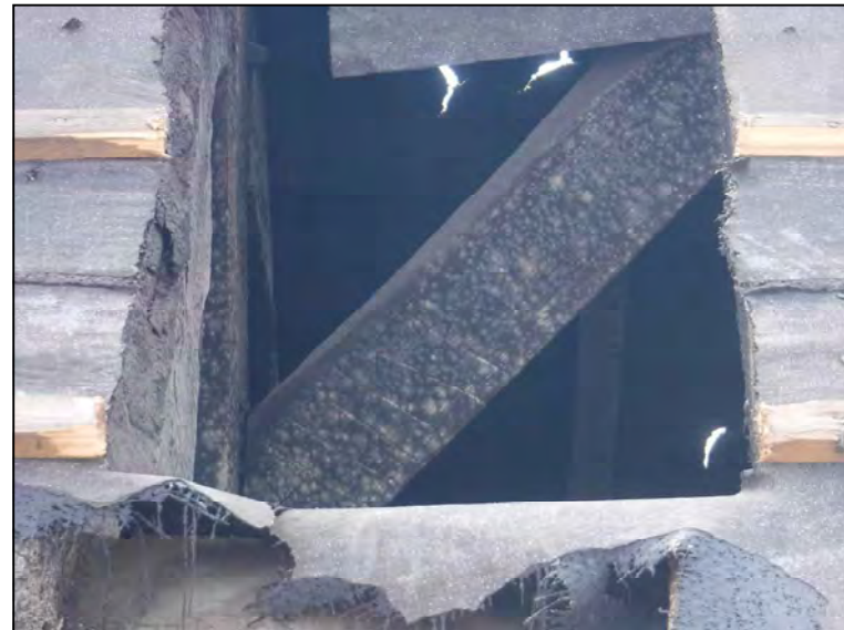
Plate 8. Diagonal brace with carpenter's mark on the southern side of Truss 3, looking east
