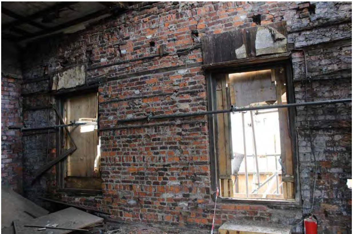
Plate 46 South range, south wall of the south side room of the first floor
