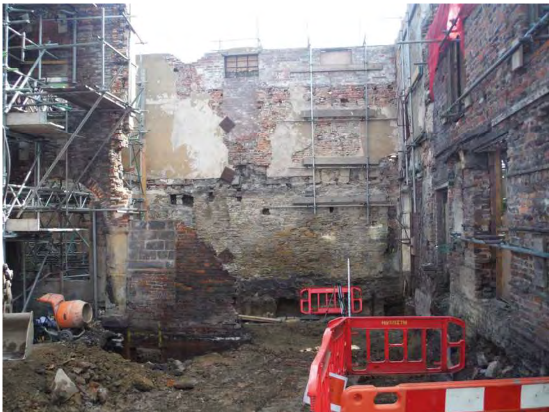
Plate 20 View of south range area during the excavation of the pile pad pits
