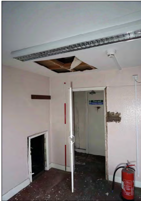
Plate 59. No. 2 second storey large room access hatch to roof space and doorway to No. 4, looking north-west
