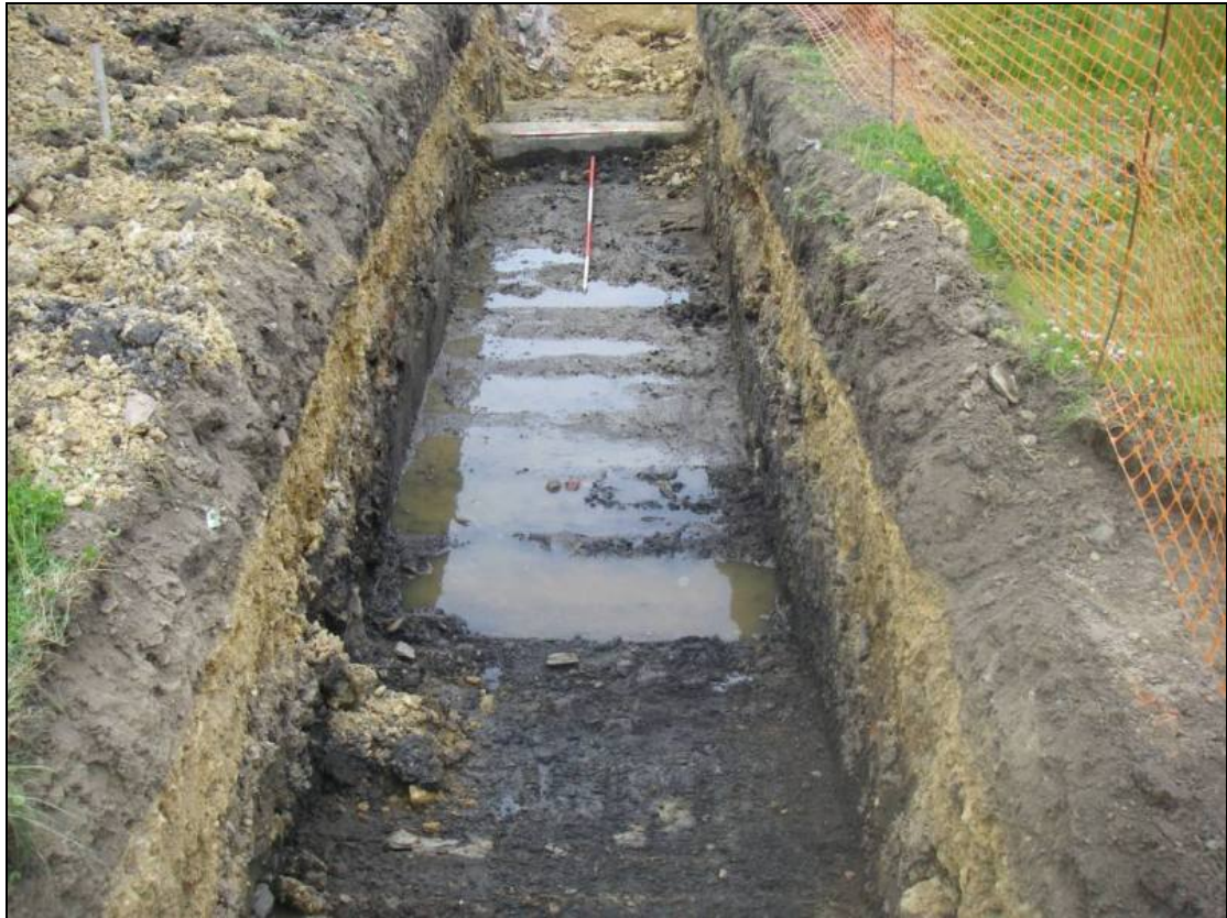
Plate 1. Ditch 115 truncated by contaminated ground, looking north
