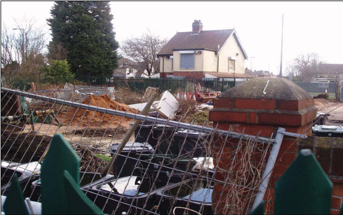
Plate 2. The enclosed yard area to the rear and western side of the site viewed facing south-east
