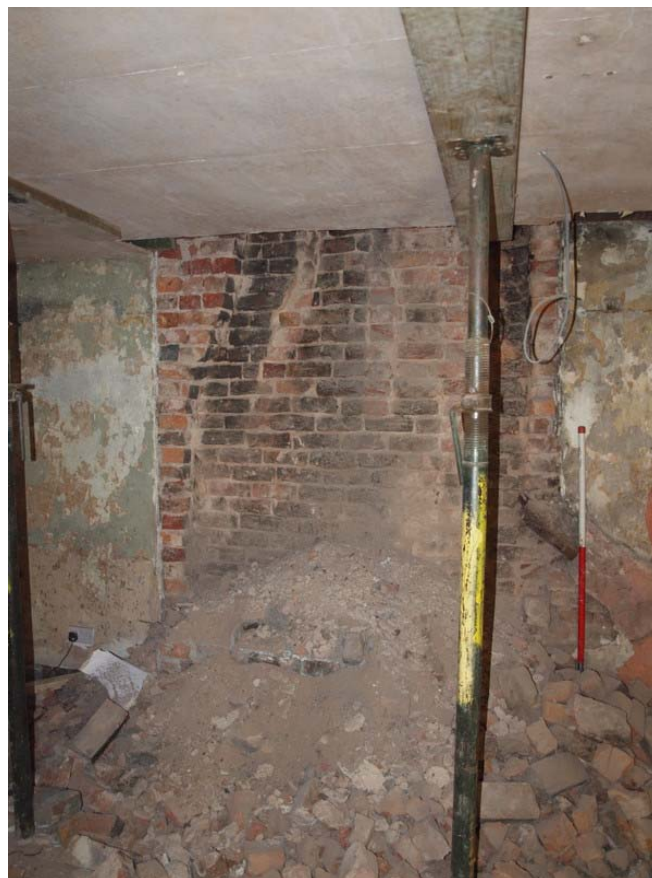
Plate 30: Chimney breast in room 6 after collapse
