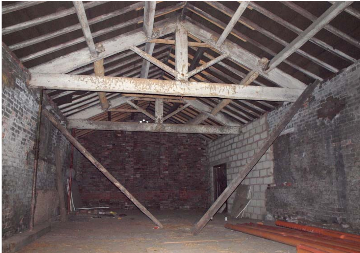
Plate 33: First floor over stable, showing king post trusses along with blocked window in west wall
